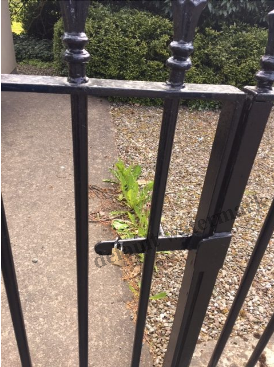
Locked pedestrian gate Lomond golf Club – reported by a reader to the LLTNPA
