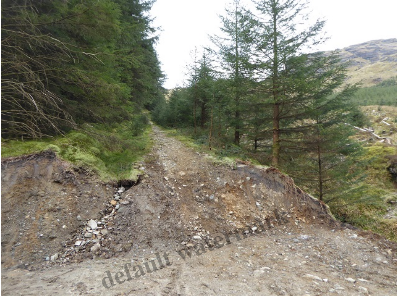
The Cowal Way, not the greatest of paths to begin with but brutally chopped off by the track extension
