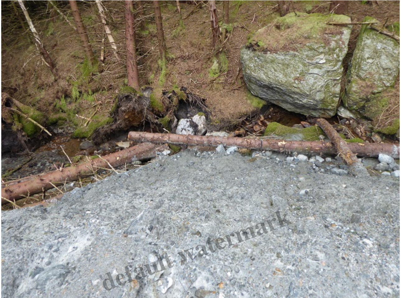
Road building material at the end of photo above shunted into the watercourse. .
