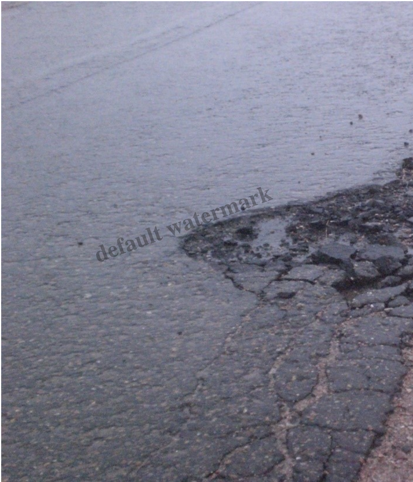
The roadway itself is crumbling away. Photo Credit Alan Bratney
