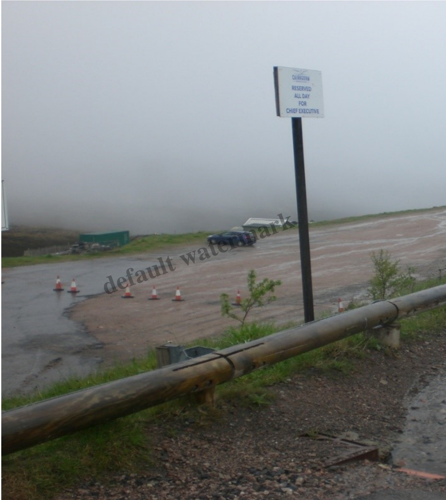
The choked/broken drain and the rainwater flowing down the car park. It's right next to the brand new
