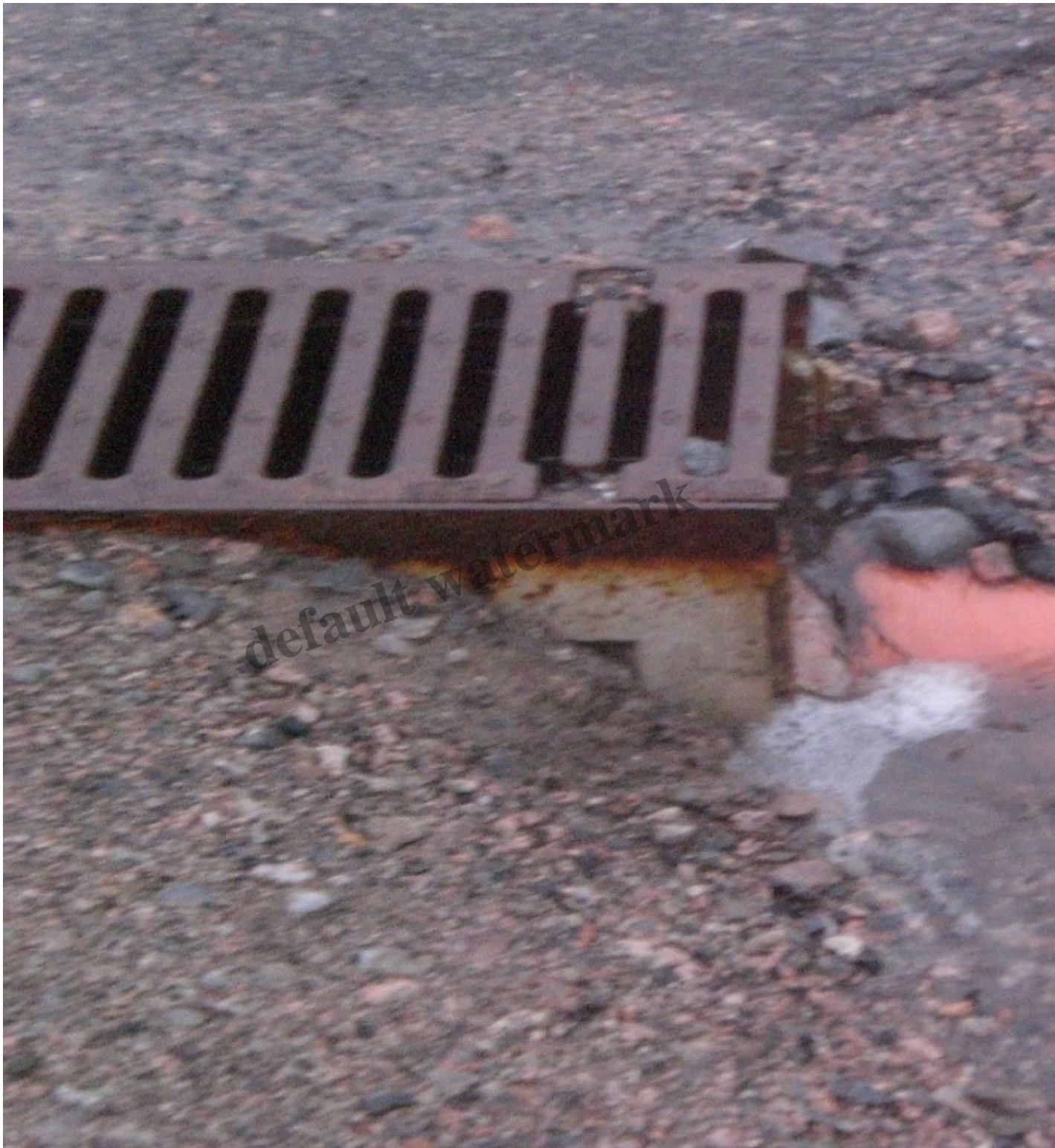
A broken/choked drain at the top of the car park. Photo Credit Alan Bratney
