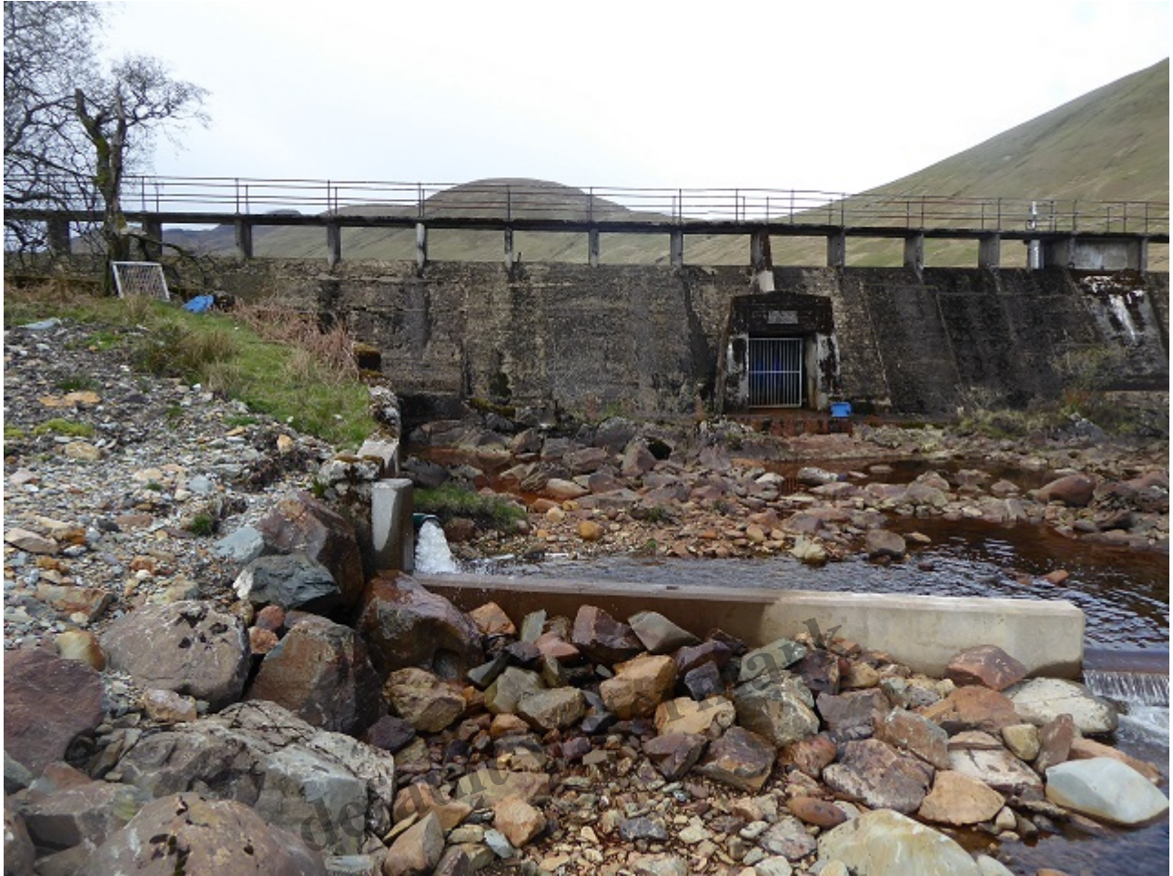
Some work had been undertaken at the new outflow below the reservoir but several apparently abandoned components were visible just below the dam
