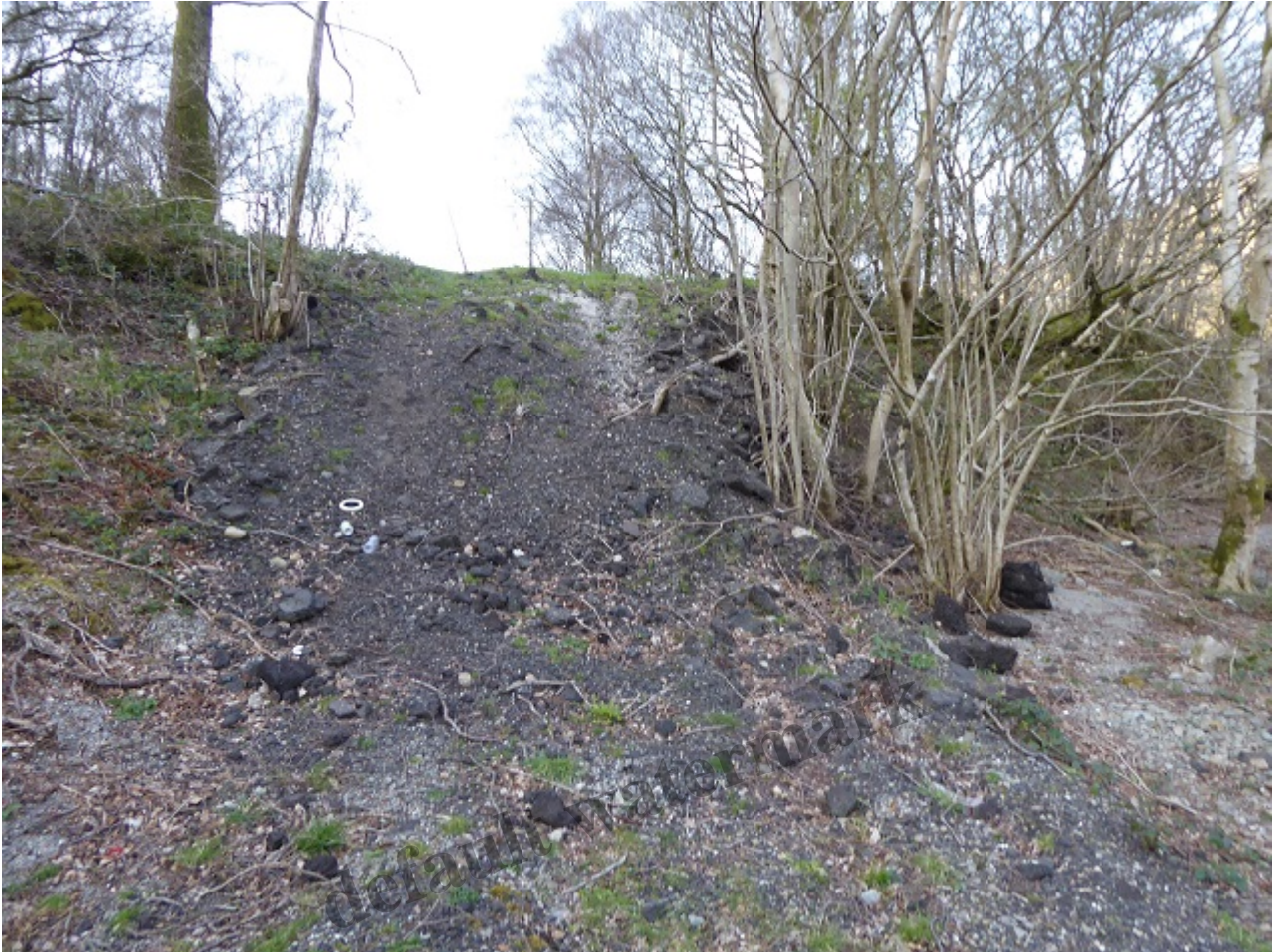
Old tarmac has been used to create a vehicle ramp down to the Loch shore to facilitate the creation of the new embankment
