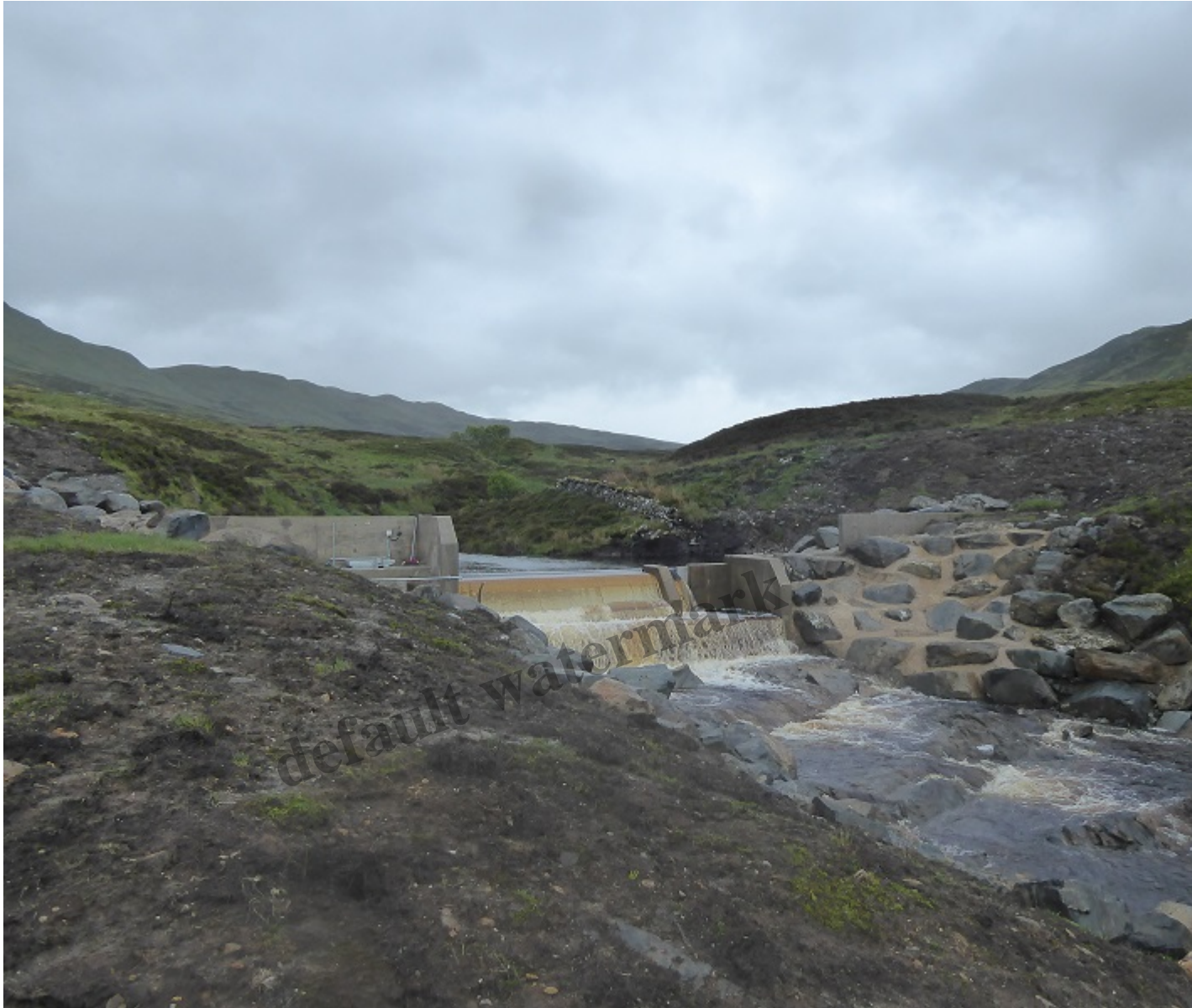
Ledcharrie hydro main intake LLTNP. Note rip rap bouldering above
