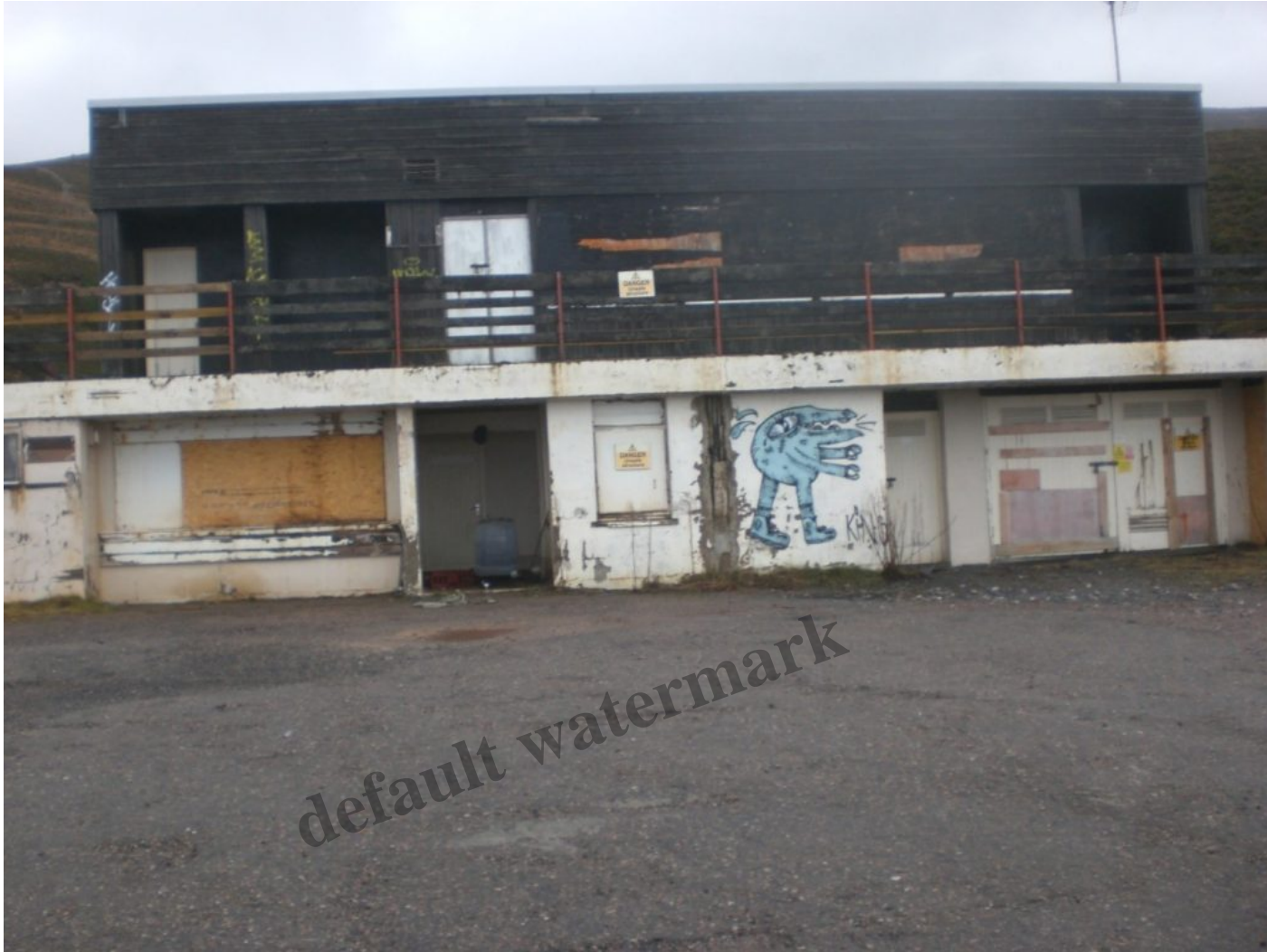
The base station with graffiti before the recent tidy up and makeover
