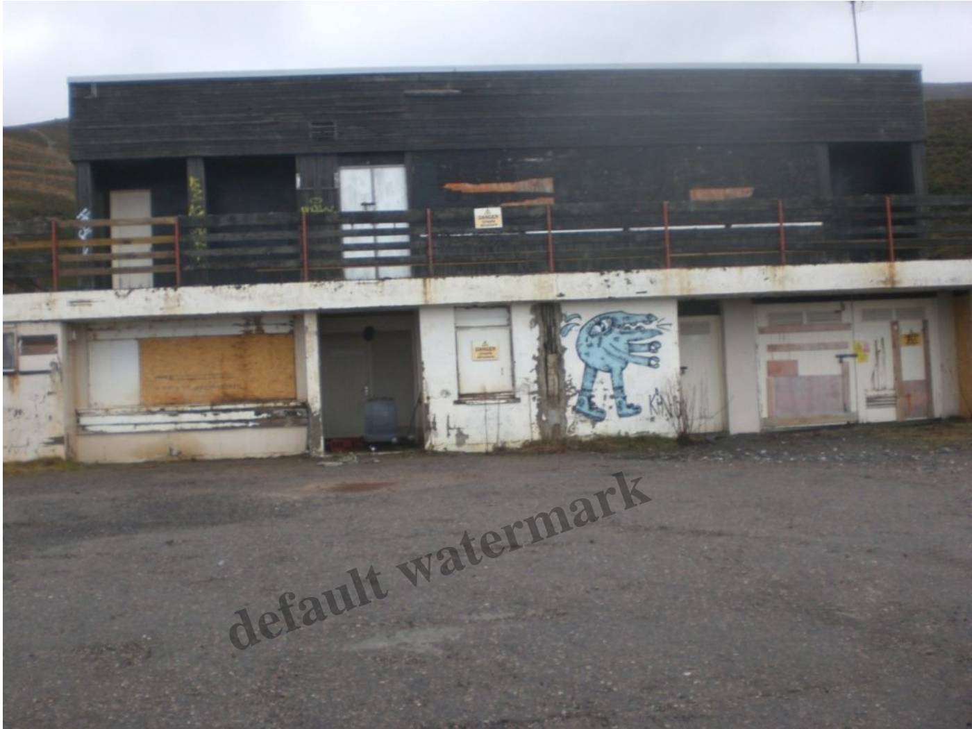
The base station with graffiti before the recent tidy up and makeover
