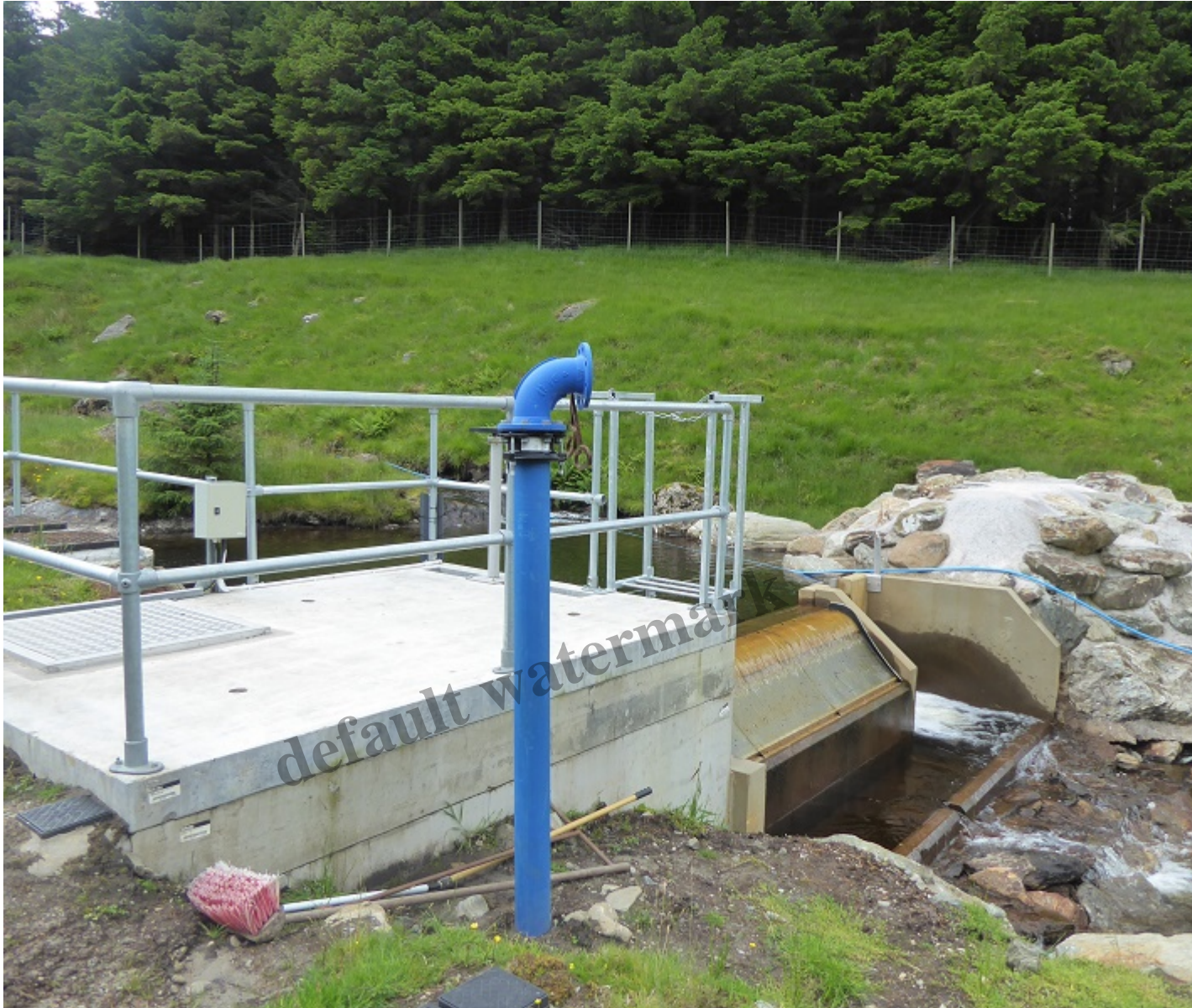
Intake on Benmore burn hydro showing how there had been some attempt to landscape far side of intake. The blue pipe is contrary to the Park's design guidance.
