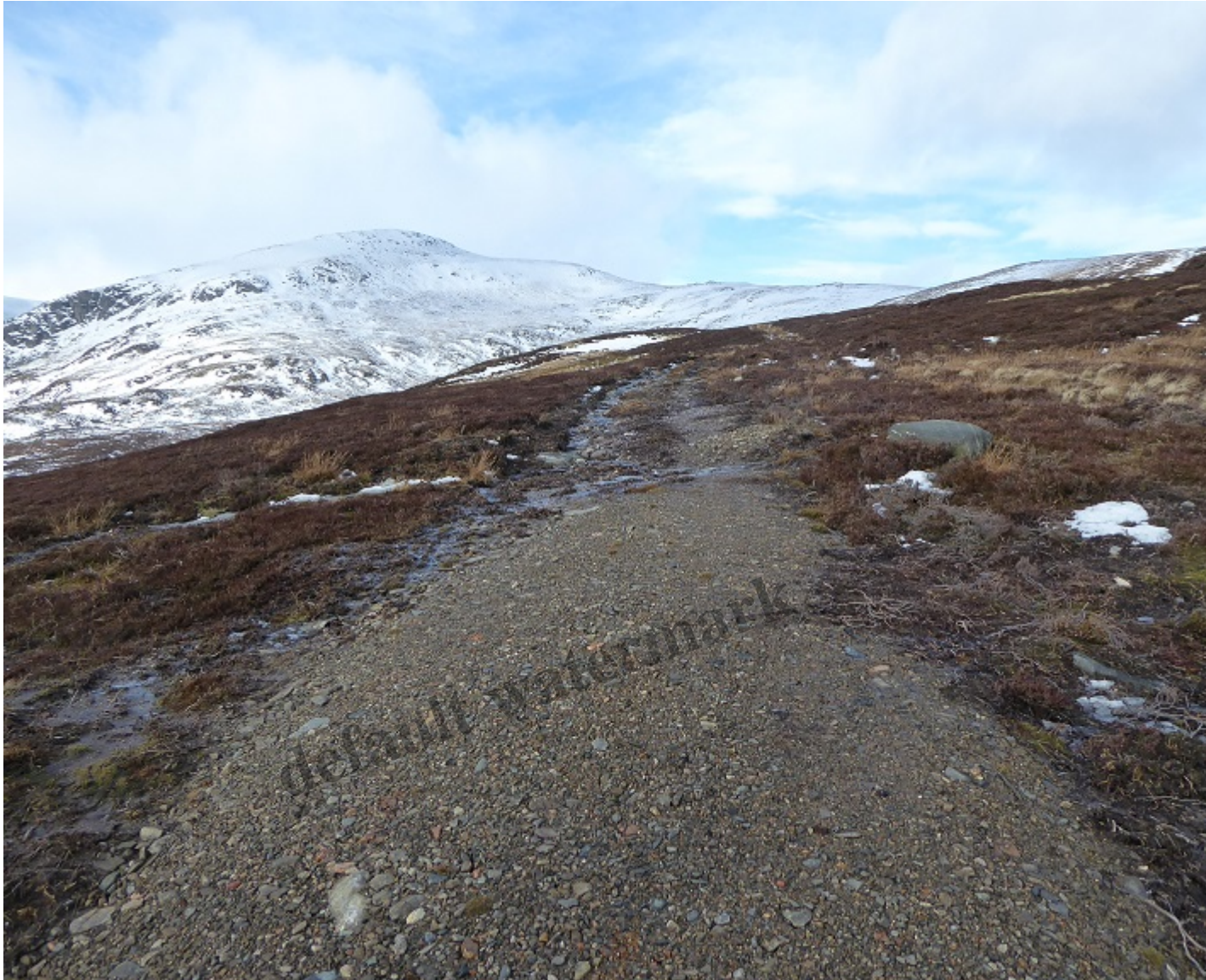
End of the new road, Mayar beyond. The landrover track continues on up towards the Mayar-Driesh
