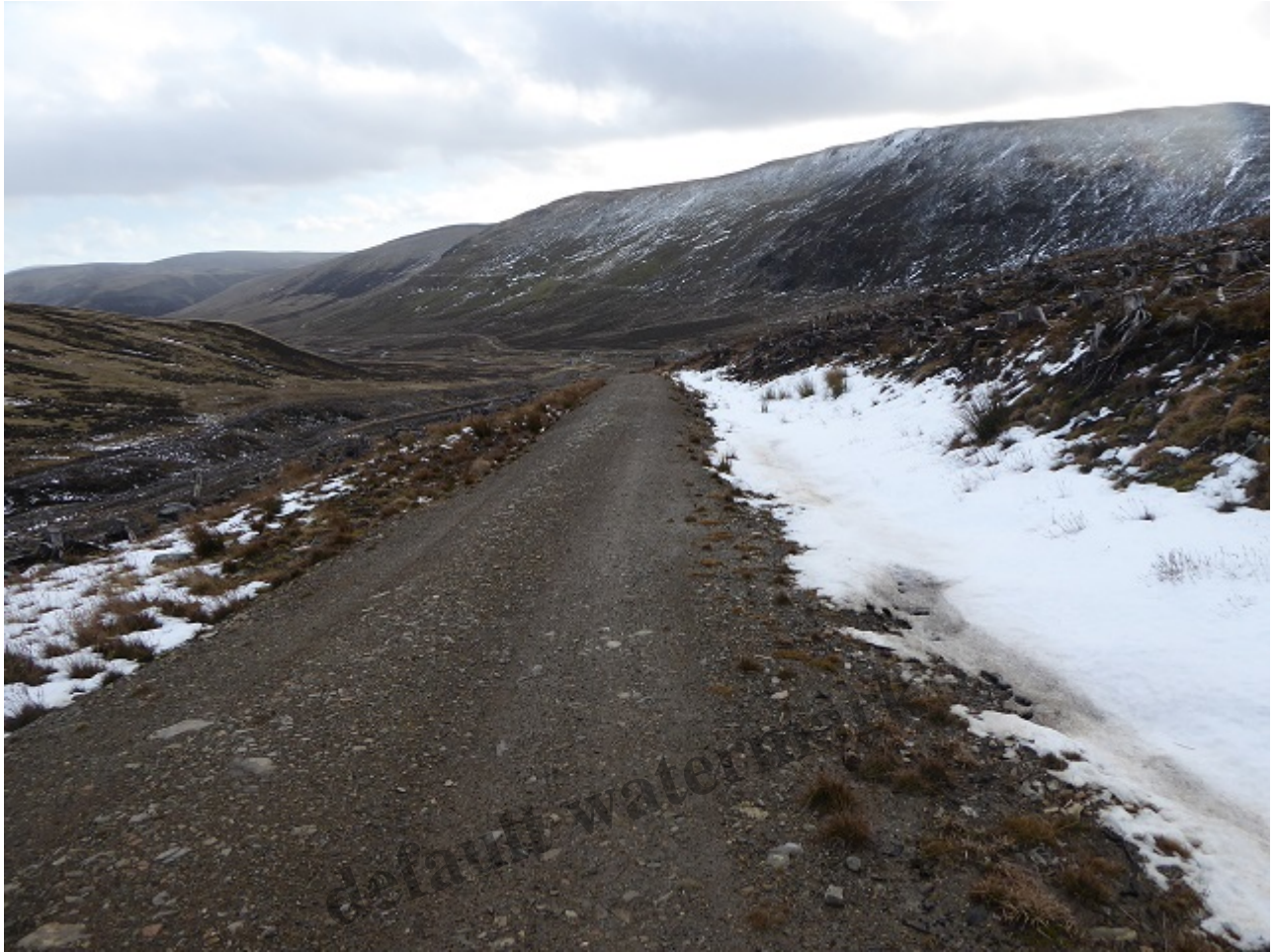
Looking down the first section of the new road, with the Kilbo hydro road visible below and two left and the old road to the head of Glen Prosen in the background beyond
