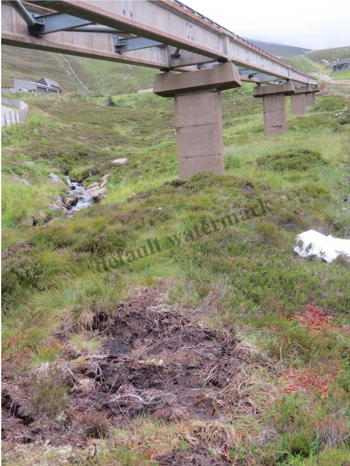
Works in 2016 took place outwith the area granted planning permission for the shieling rope tow and close to the funicular
