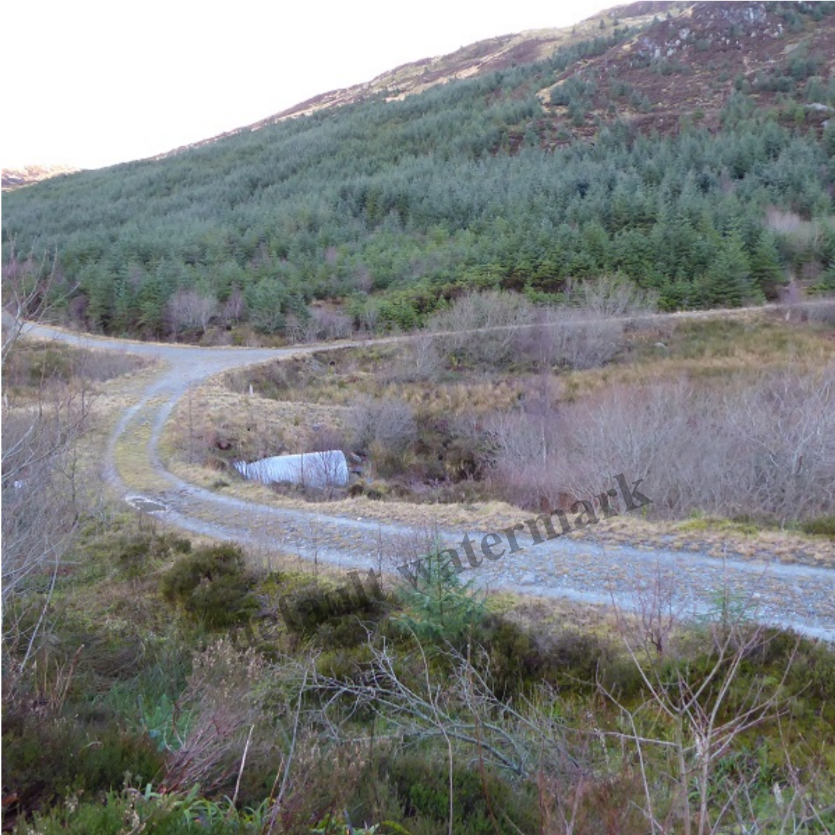
Forestry culvert under the track just below the intake – the hydro pipe lies under the line of rush just behind.
