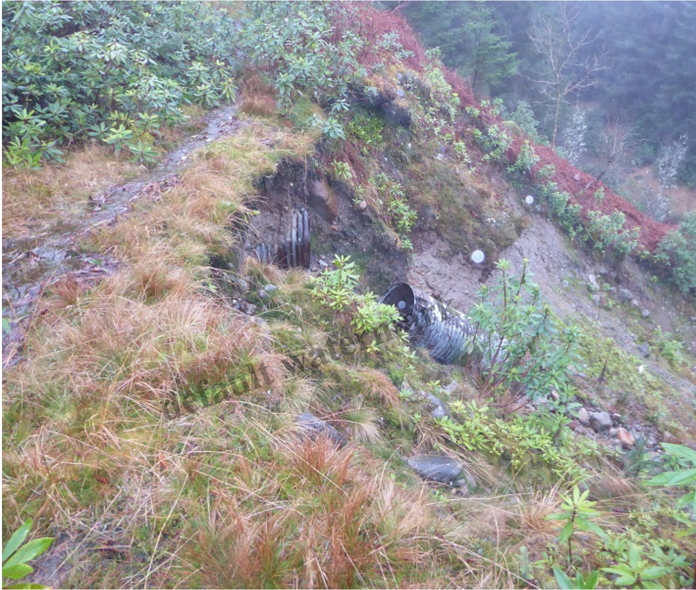
Section of track which had collapsed and fallen into the river
