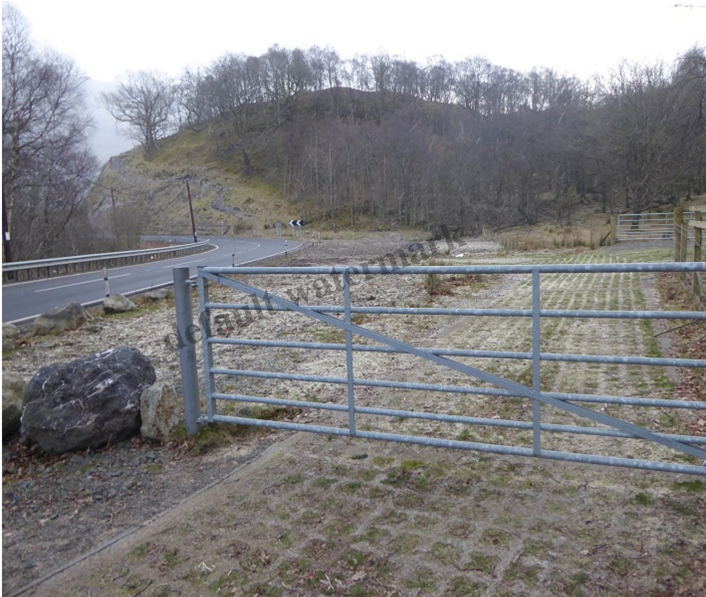
Access to pulpit Rock by the section of upgraded A82 with metal netting visible on cutting behind (see below)
