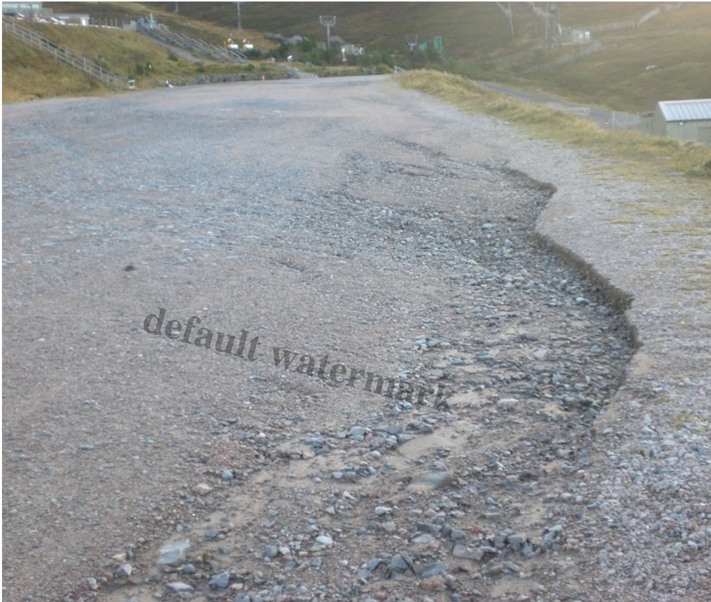
Half the lower car park has been eroded by the flooding from the blocked drainage ditch. Photo Credit: Creag Bratney November 2018.
