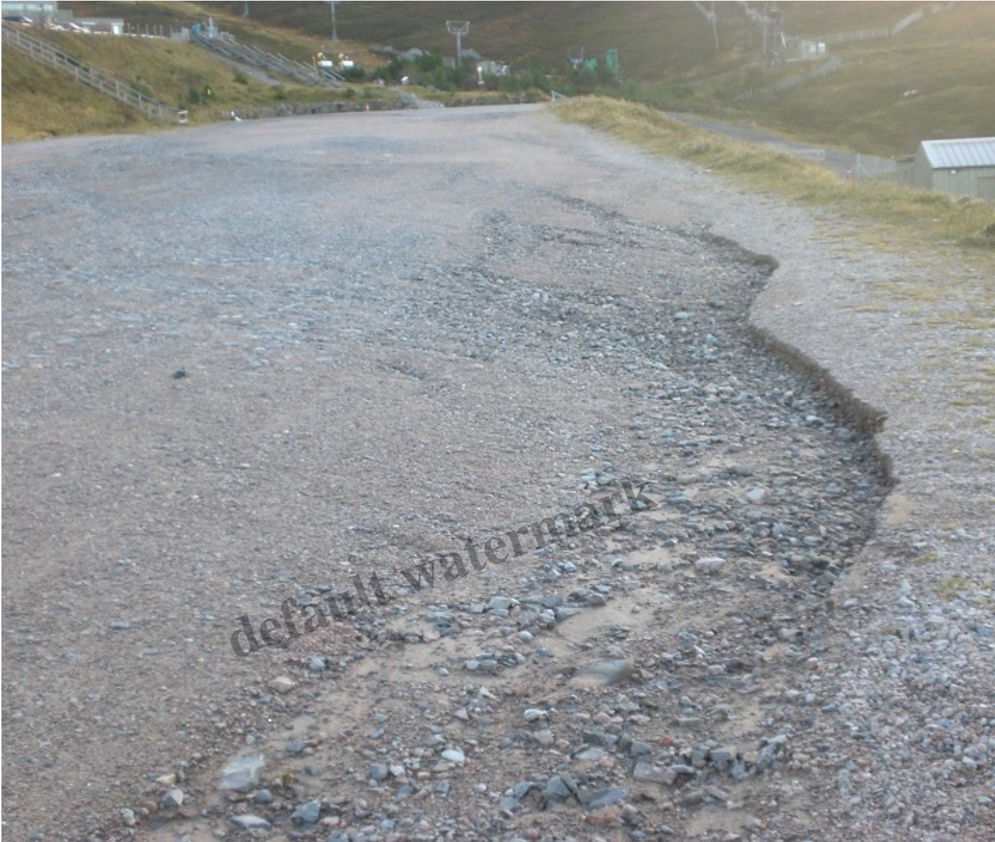
Half the lower car park has been eroded by the flooding from the blocked drainage ditch. Photo Credit: Creag Bratney November 2018.
