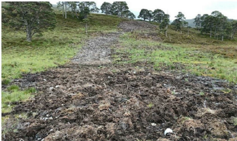
Figure 3.8 A restored pipe trench, this one in the Glen Affric National Scenic Area and Strathglass Complex SAC, shortly after it was backfilled and the surface restored. Once vegetation is established on the bare peat the pipe route will be completely invisible.
