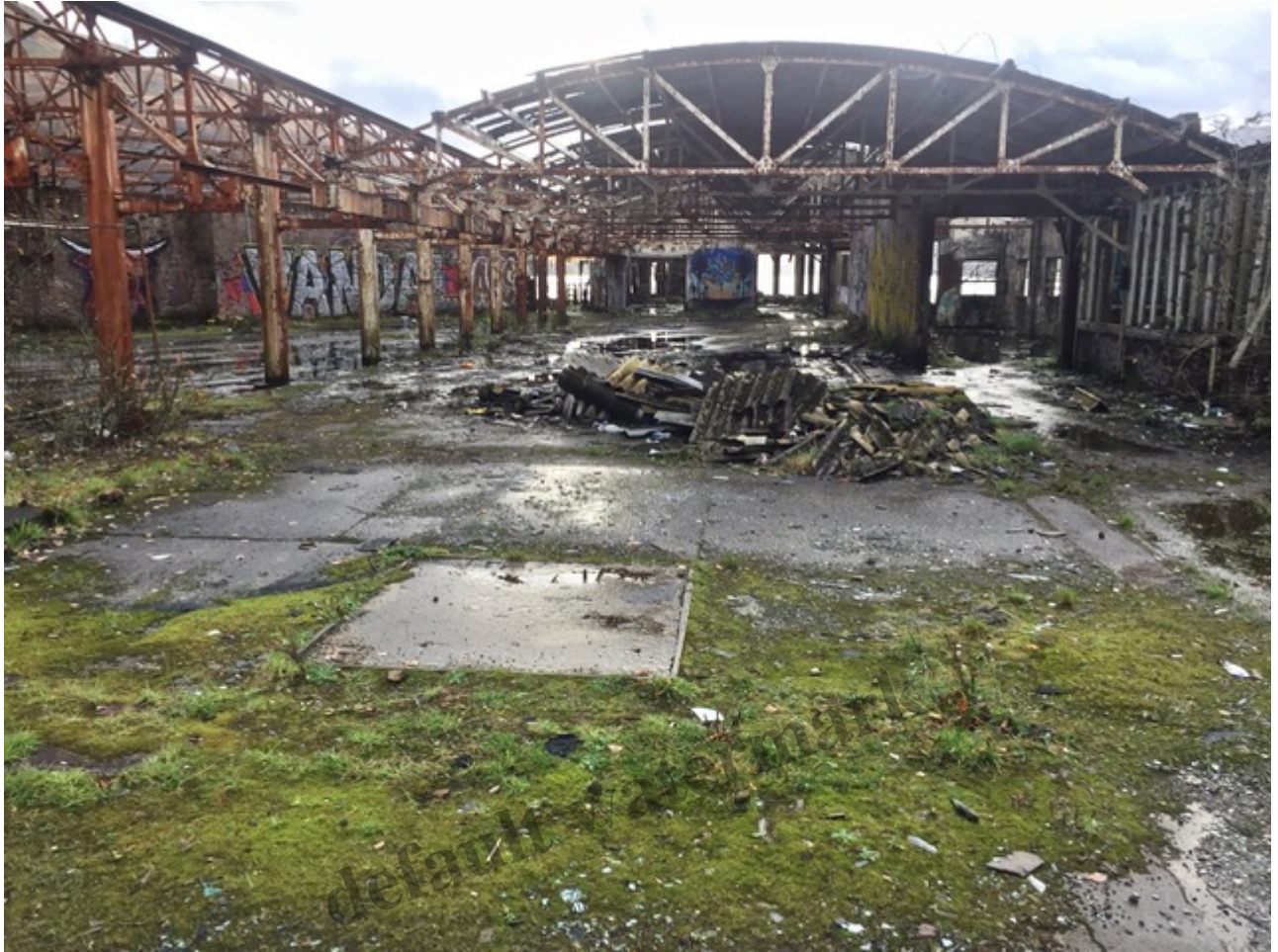
The derelict structures on the concrete platform by the shore of Loch Long cover an extensive area Photo Credit Nick Halls
