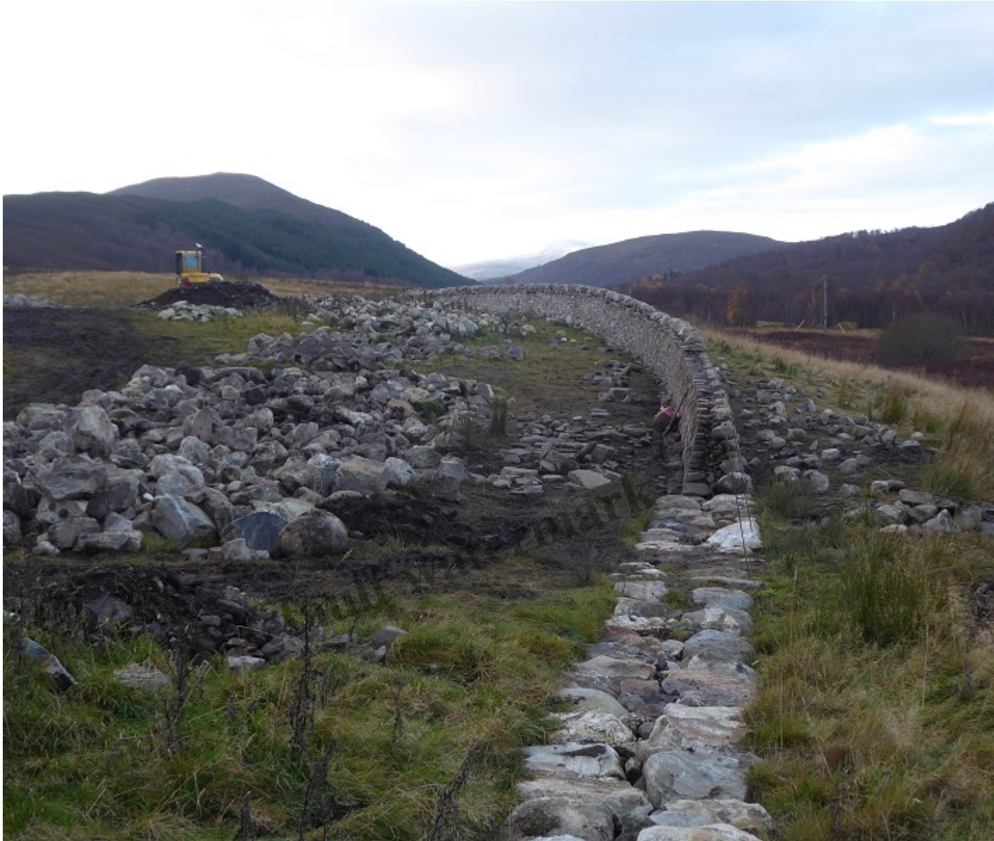
Dry stane wall building in Glen Tromie by Killiehuntly Oct 2017 – such landscaping work supports local employment
