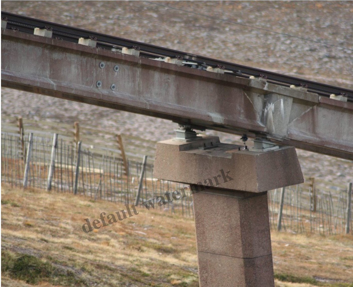
Monitoring device at tunnel mouth – note the apparent cracks in the t-section above. Photo credit Te
