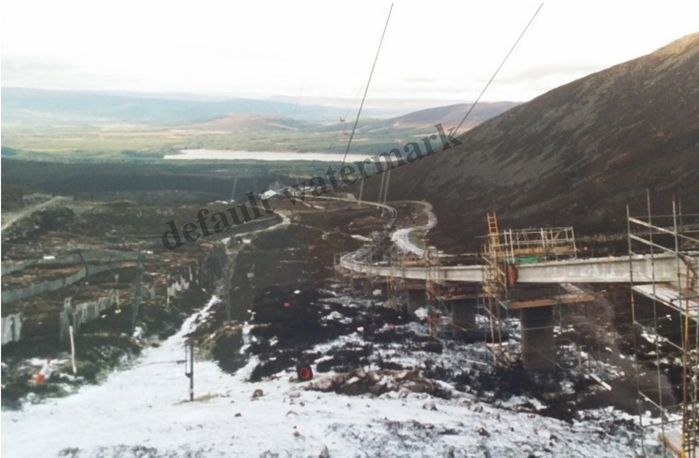
Construction was carried out with very little ground damage. Photo credit George Paton.
