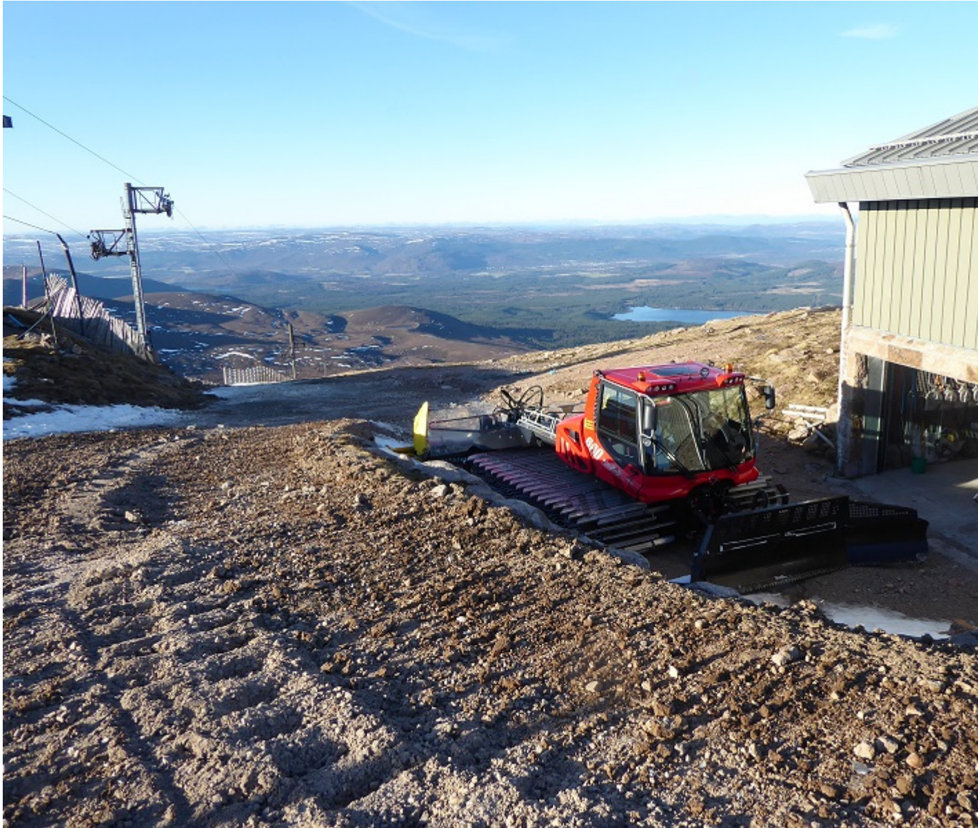
The damage to the ground around the Ptarmigan is extensive
