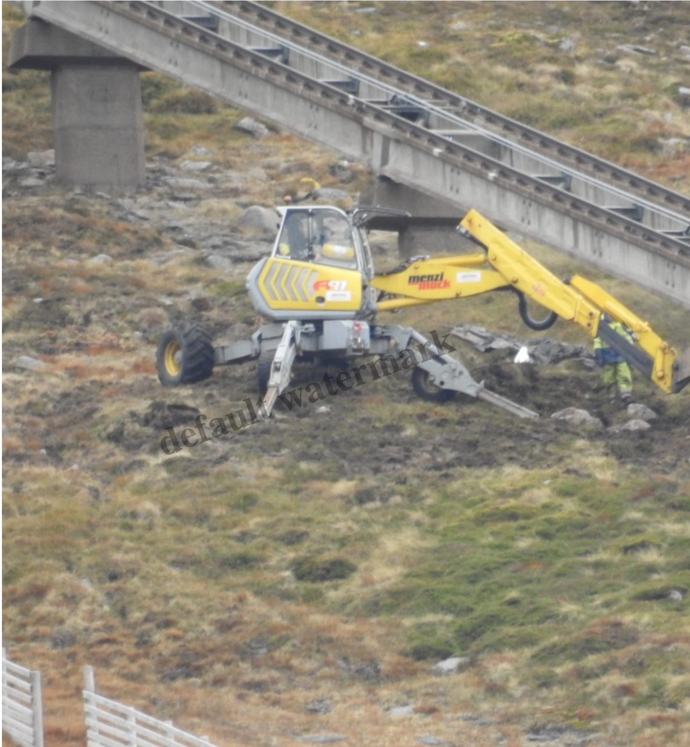
Digger excavating one of the shoogly pillars 18th October (apparently the pillar below the one in the measures being taken to protect the ground. Photo Credit Gus Jones
