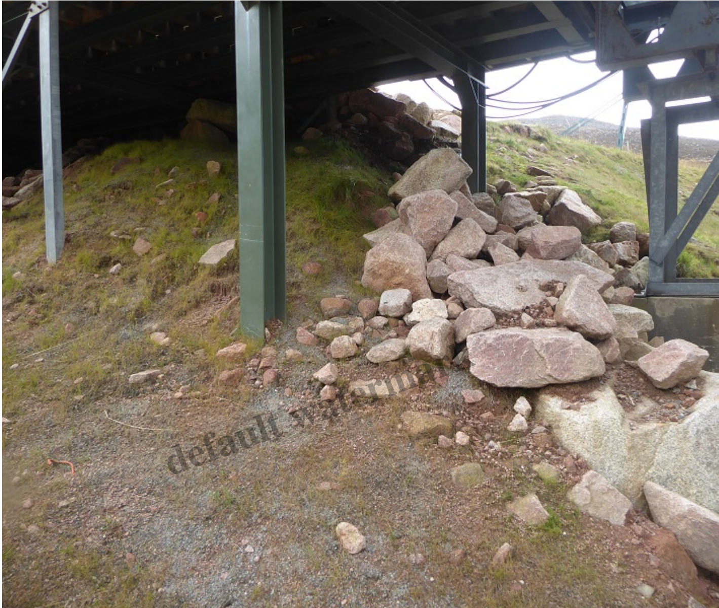
Boulders under the Coire Cas gantry – dumped there after emergency work to save the gantry from
