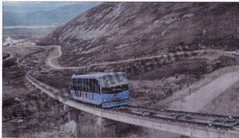
One of the concrete beams that carries the 2km funicular track has been found to have a crack in it, with fears that all 94 pairs on the route could be affected.
