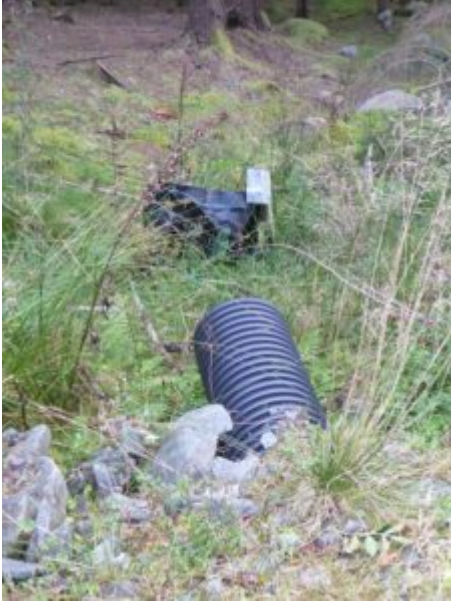
Protruding culvert on new section access track
