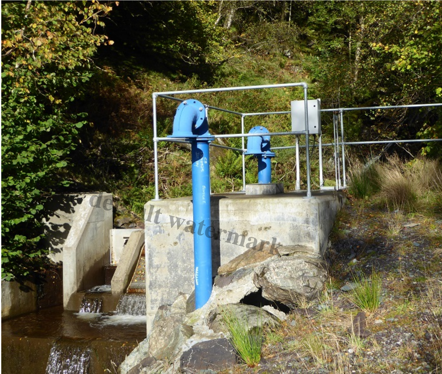
More blue pipes and bare concrete structures
