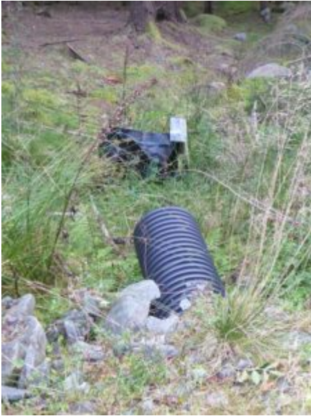
Protruding culvert on new section access track
