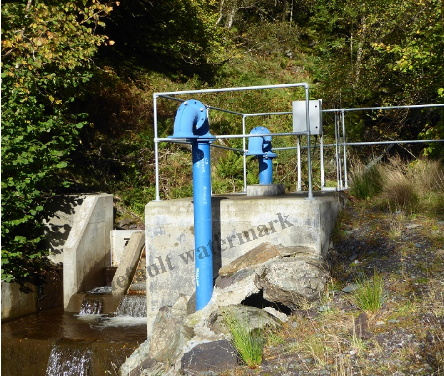
More blue pipes and bare concrete structures
