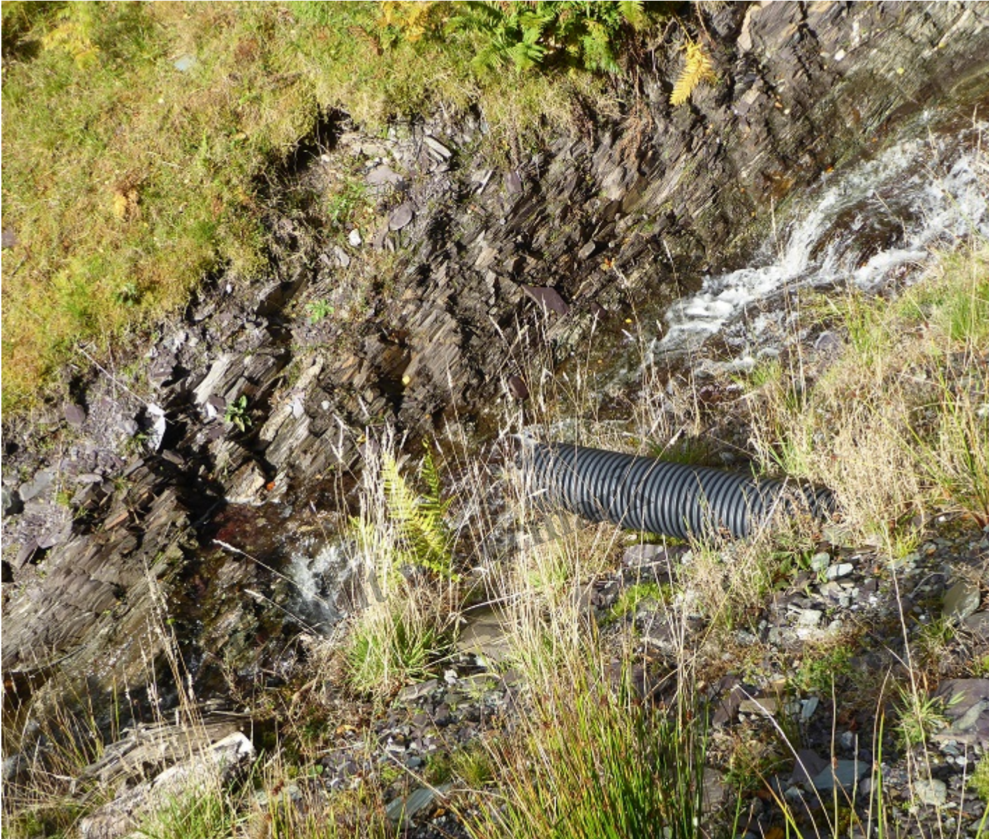
The seemingly inevitable protruding culvert – this one just below the intake
