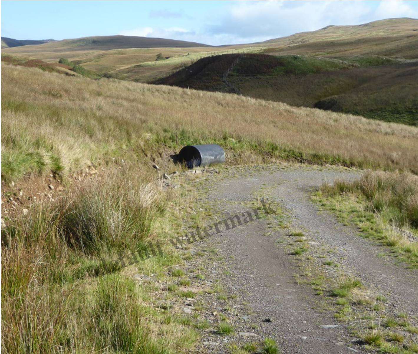
Pipe being used as a drain on access road to power house
