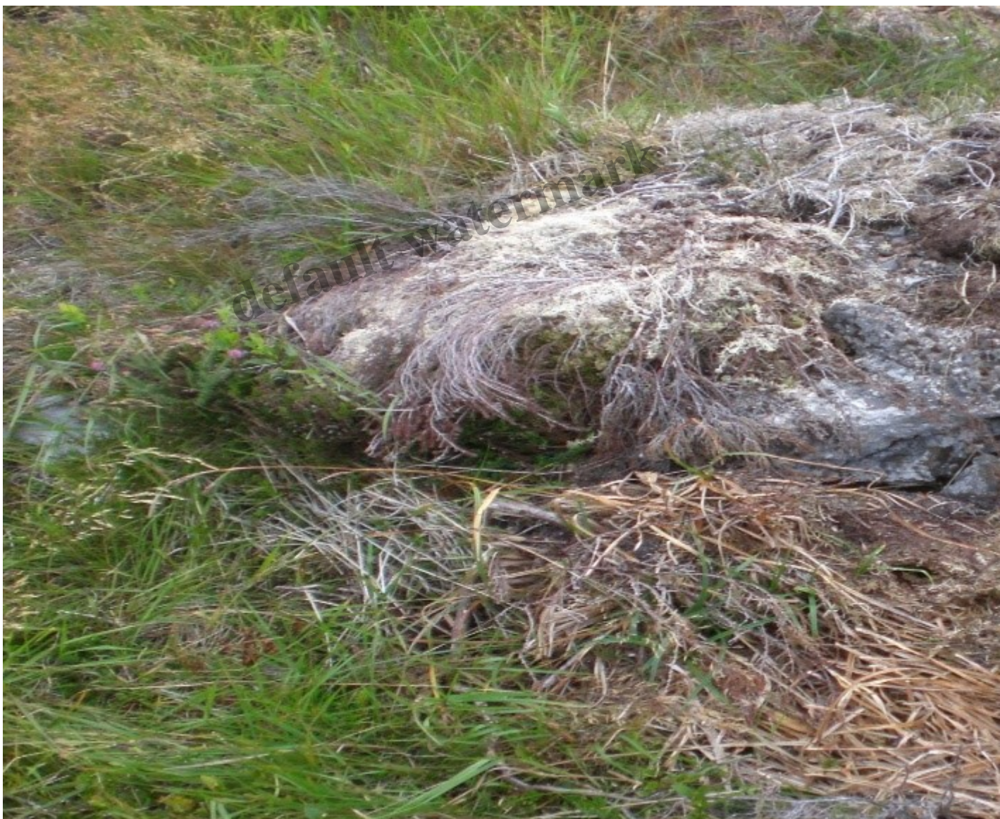
Exposed concrete which has not been broken out to 200mm below surface. Photo Credit Alan Bratt
