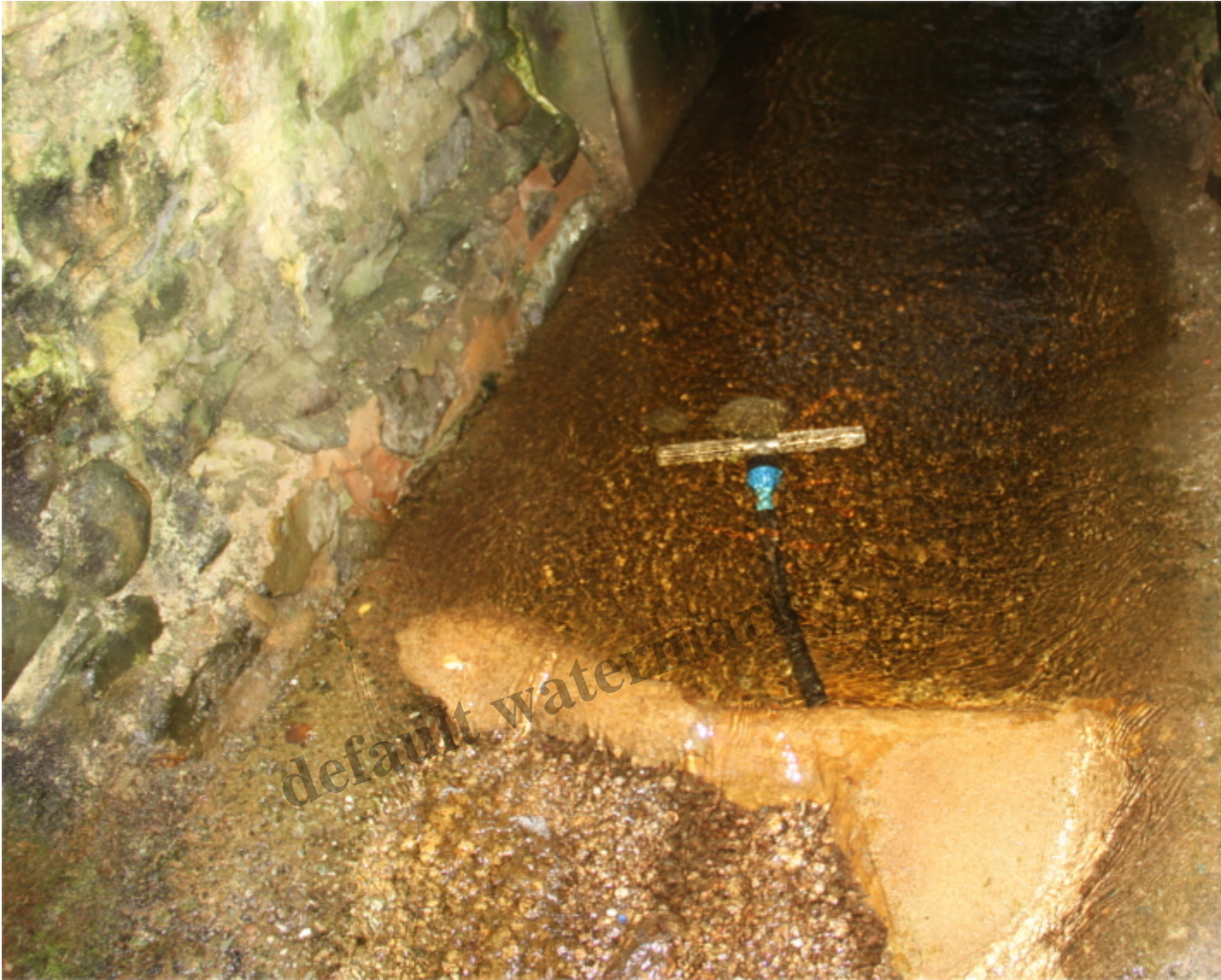
The upgraded water intake under the road bridge – photo credit Ross MacBeath
