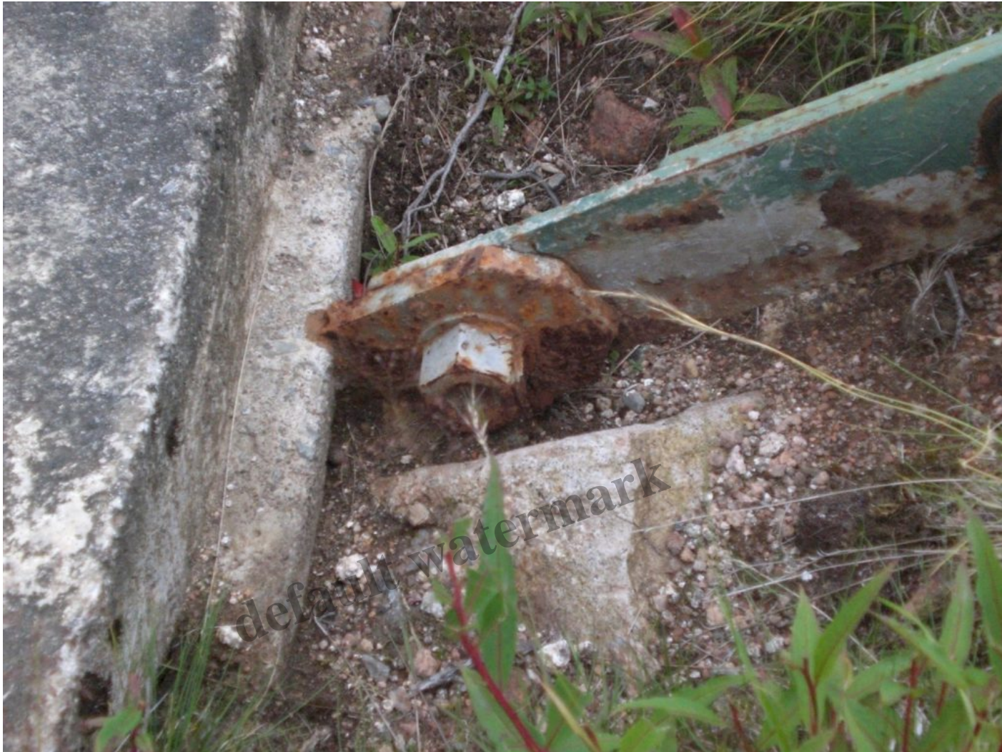
“Buried mild steel parts should be exposed and protected” – photo credit Alan Bratley
