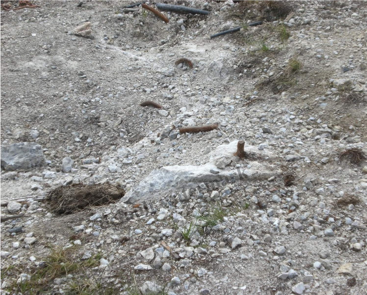
Very dangerous reinforcing metal rods that have been left protruding from the concrete.
