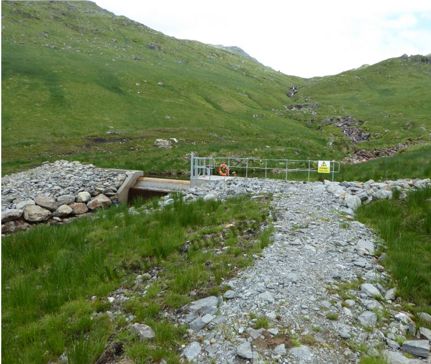
The main intake on the Allt a Chuillinn hydro scheme looking up towards Coire a Chuillinn which forms a designated Wild Land Area
