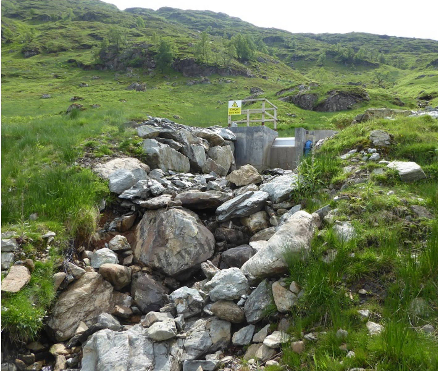
Below the third intake, blue pipe, warning signs and all – the burn started flowing again in bottom left
