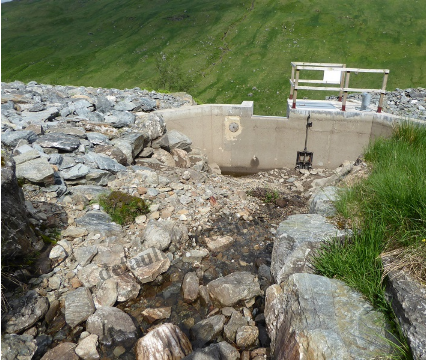
The third intake from above with flowing water visible in the foreground
