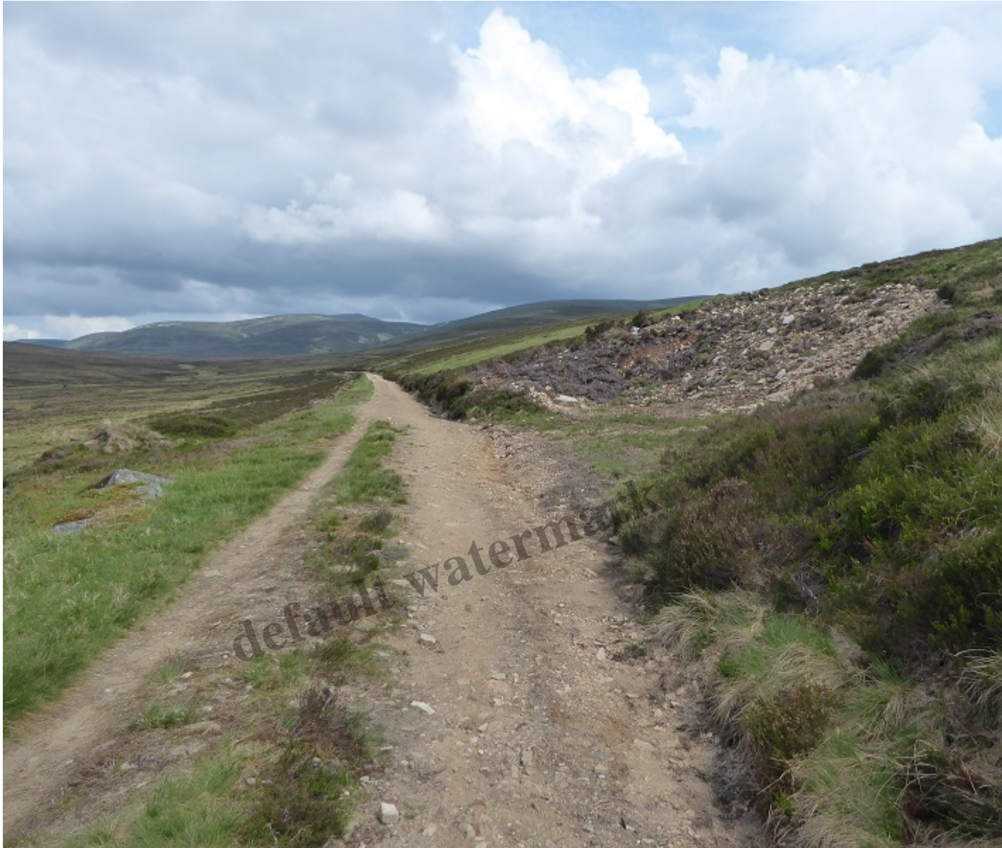
The start of the first section of upgraded track, with newly worked borrow pit on right
