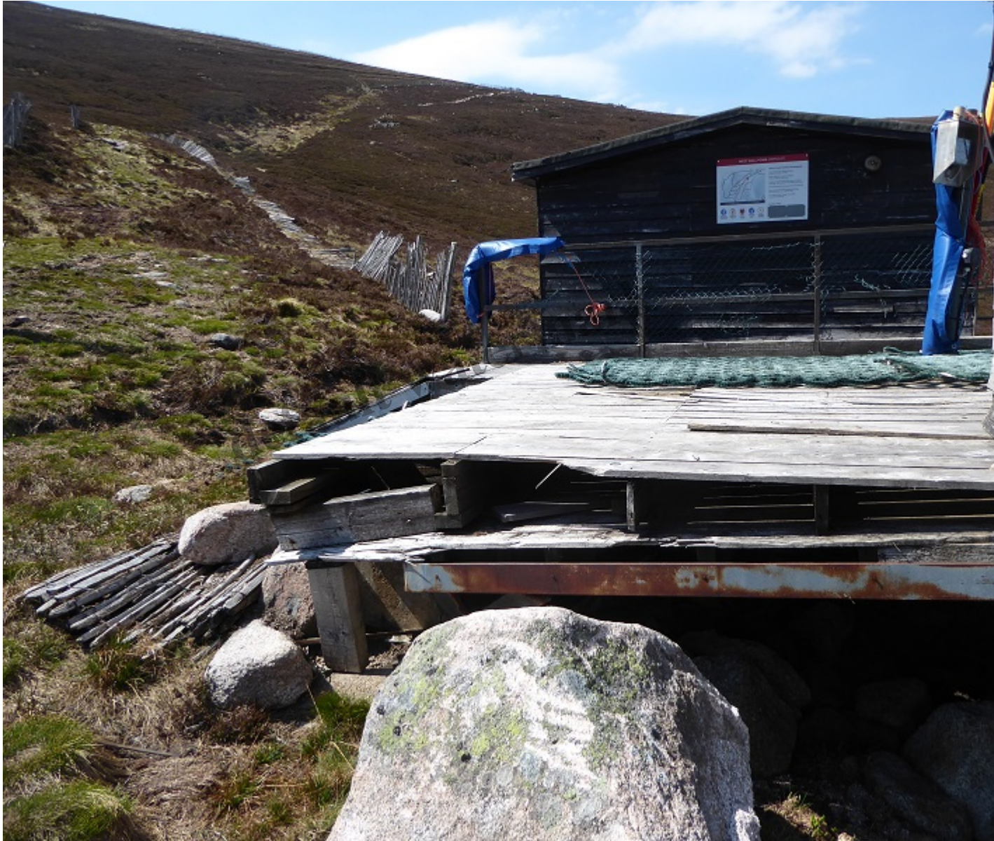
The West Wall poma base, in urgent need of repair, with electricity sub-station and collapsed snow fence behind on 26th May 2018
