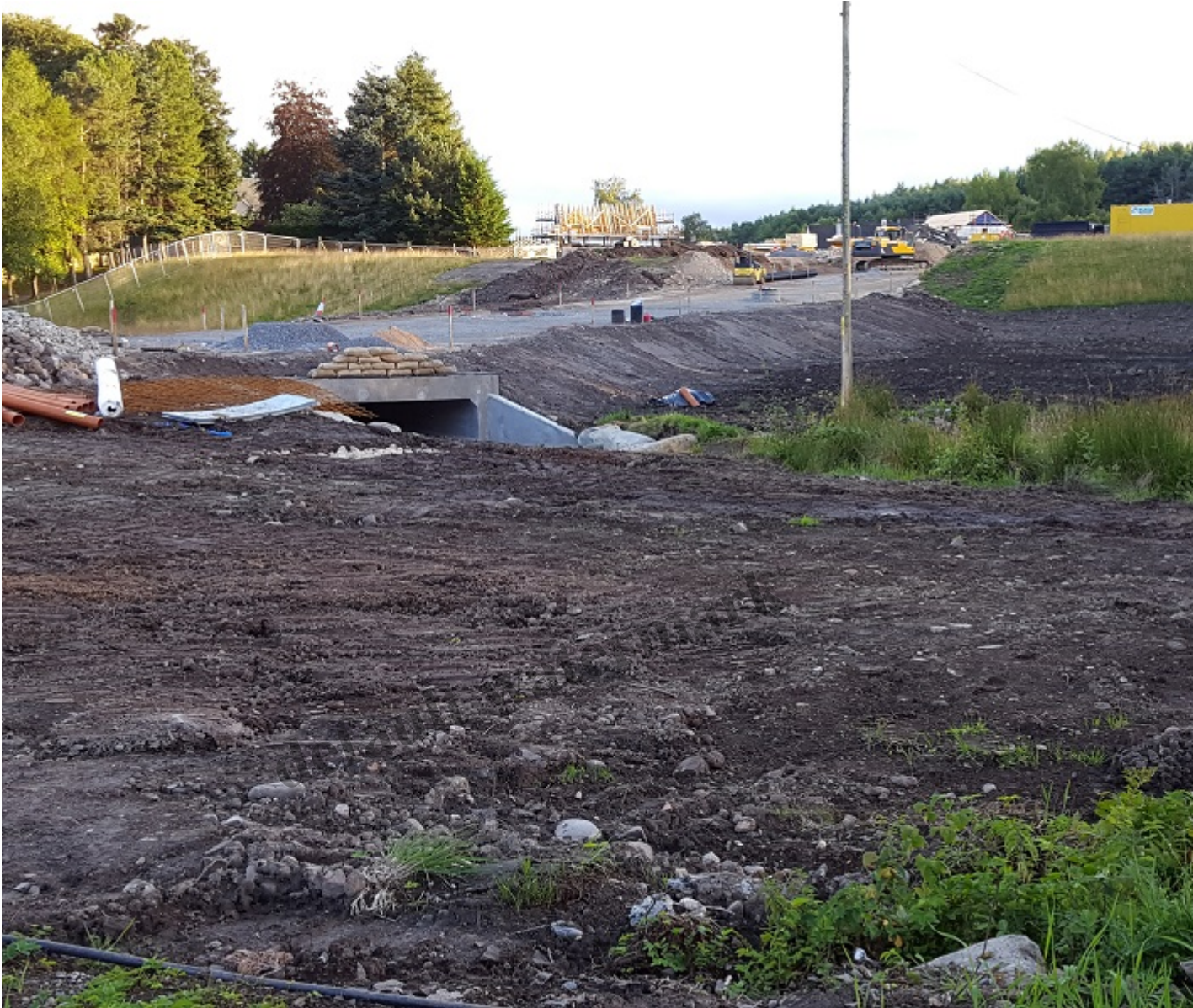
Photo 11 Virtually all of this rich wetland destroyed and levels raised with soil fill (August 2017)
