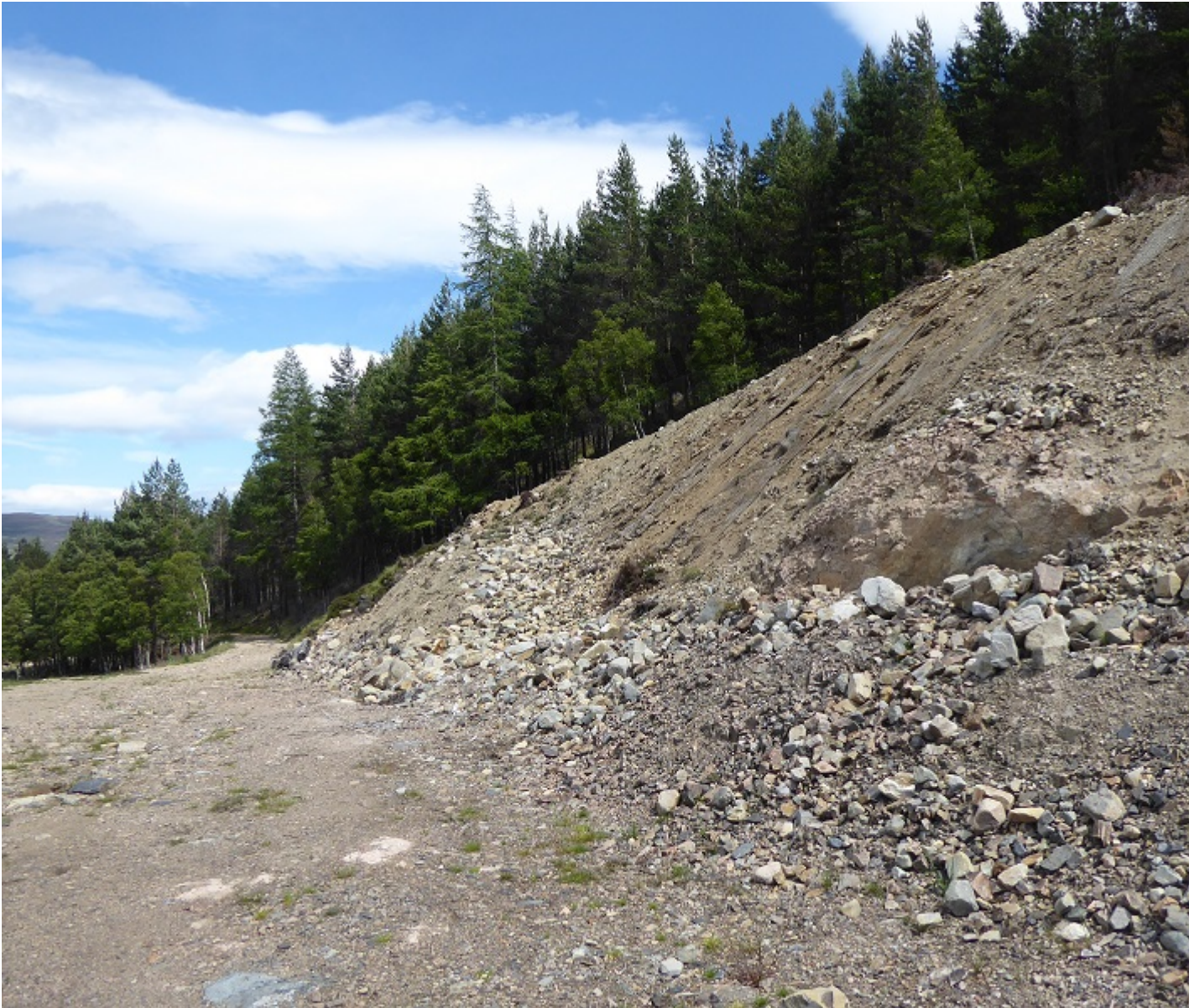
The slope by the main Corriemulzie intake in July 2017 – note how the geotextile, centre, has failed the slope and the wide area for vehicle use below
