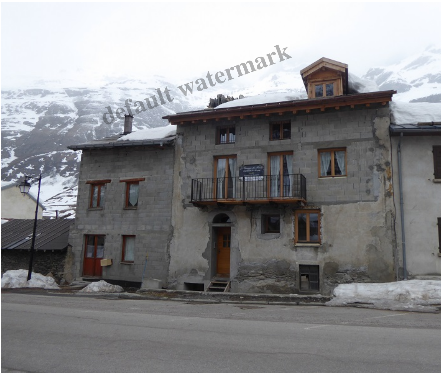
Unfinished building renovation/extension Bessans – note how concrete masonry blocks have been a
