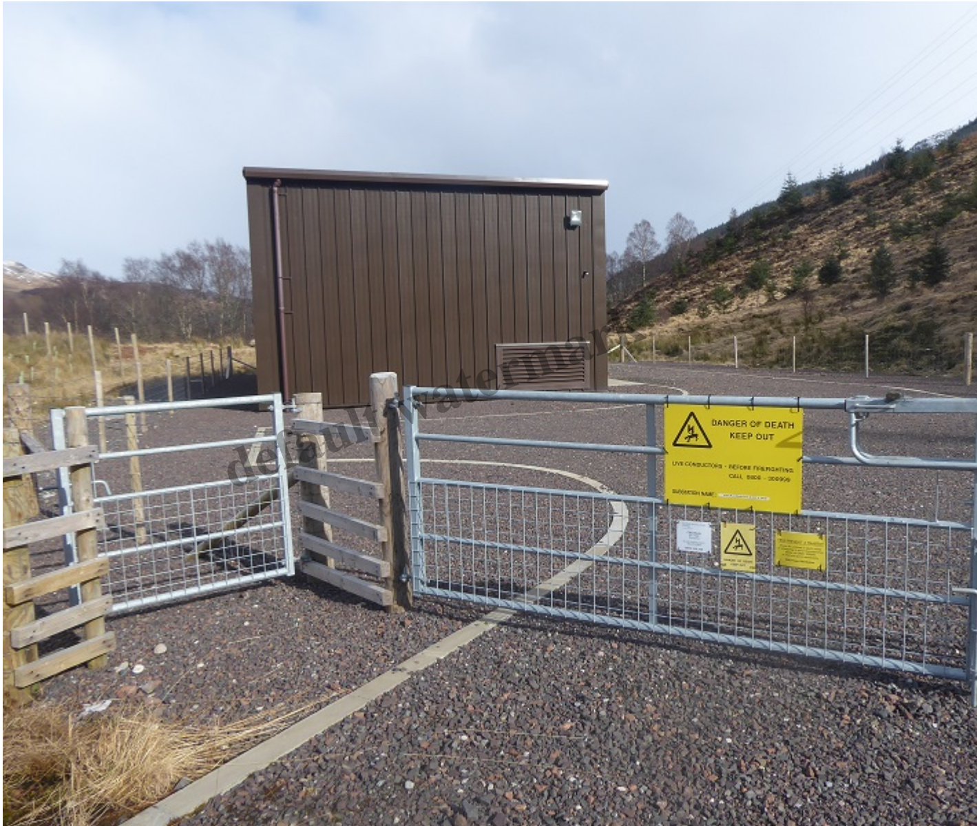
New electricity sub-station just above the main road in Glen Dochart, at the start of the main Allt Chaoirach track
