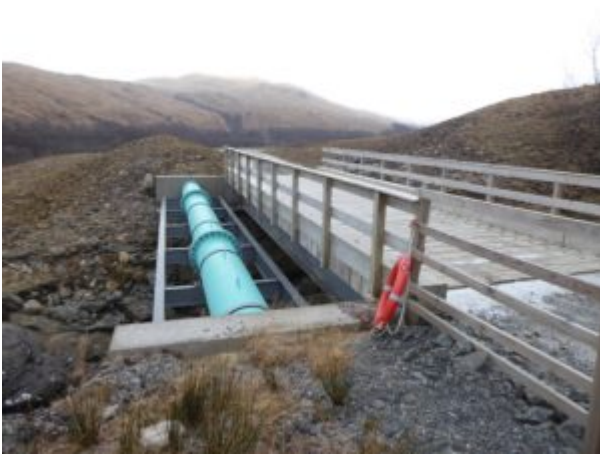
Allt Chuilinn penstock – according to Park guidance this should have been hidden UNDER the bridge
