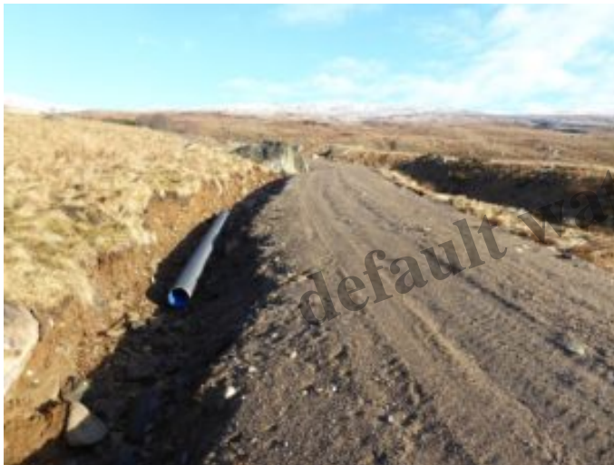
Poorly constructed ditch and abandoned? section of pipe
