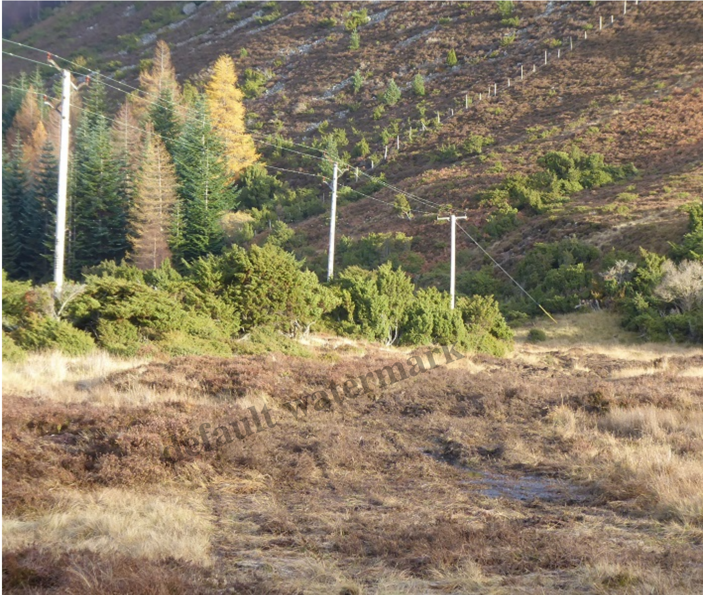
The new powerline, which lies beneath the vehicle track starting bottom centre, will replace the pylor
