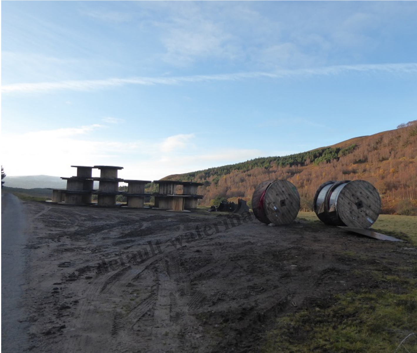
Evidence of the amount of new electric cable which has been undergrounded
