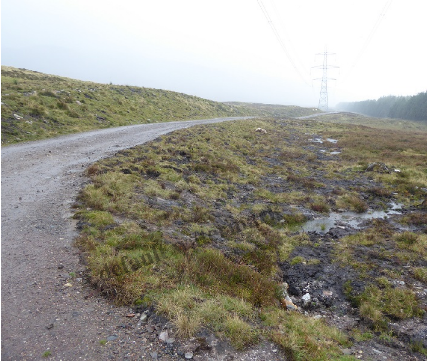
The northernmost end of the track. Note how the low angle of the embankment above the track has vegetation to recover quickly while stored turfs have been effectively used to restore the ground below track. October 2017.
