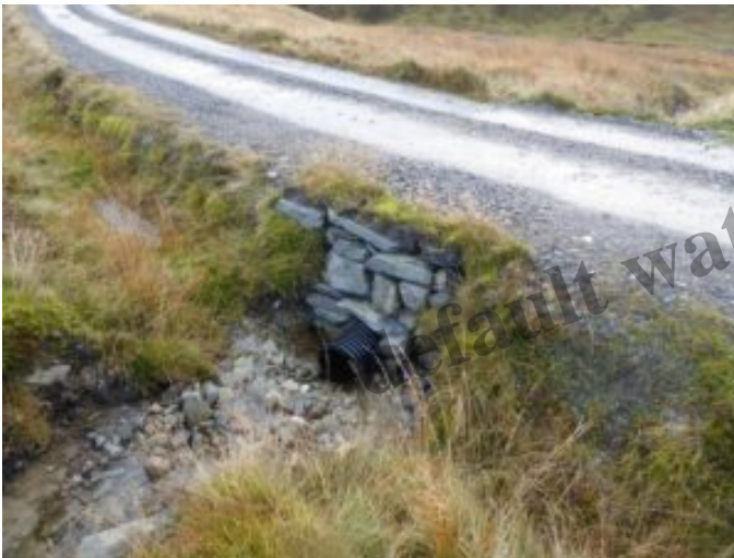
Same culvert, other side of road, protruding – why?
