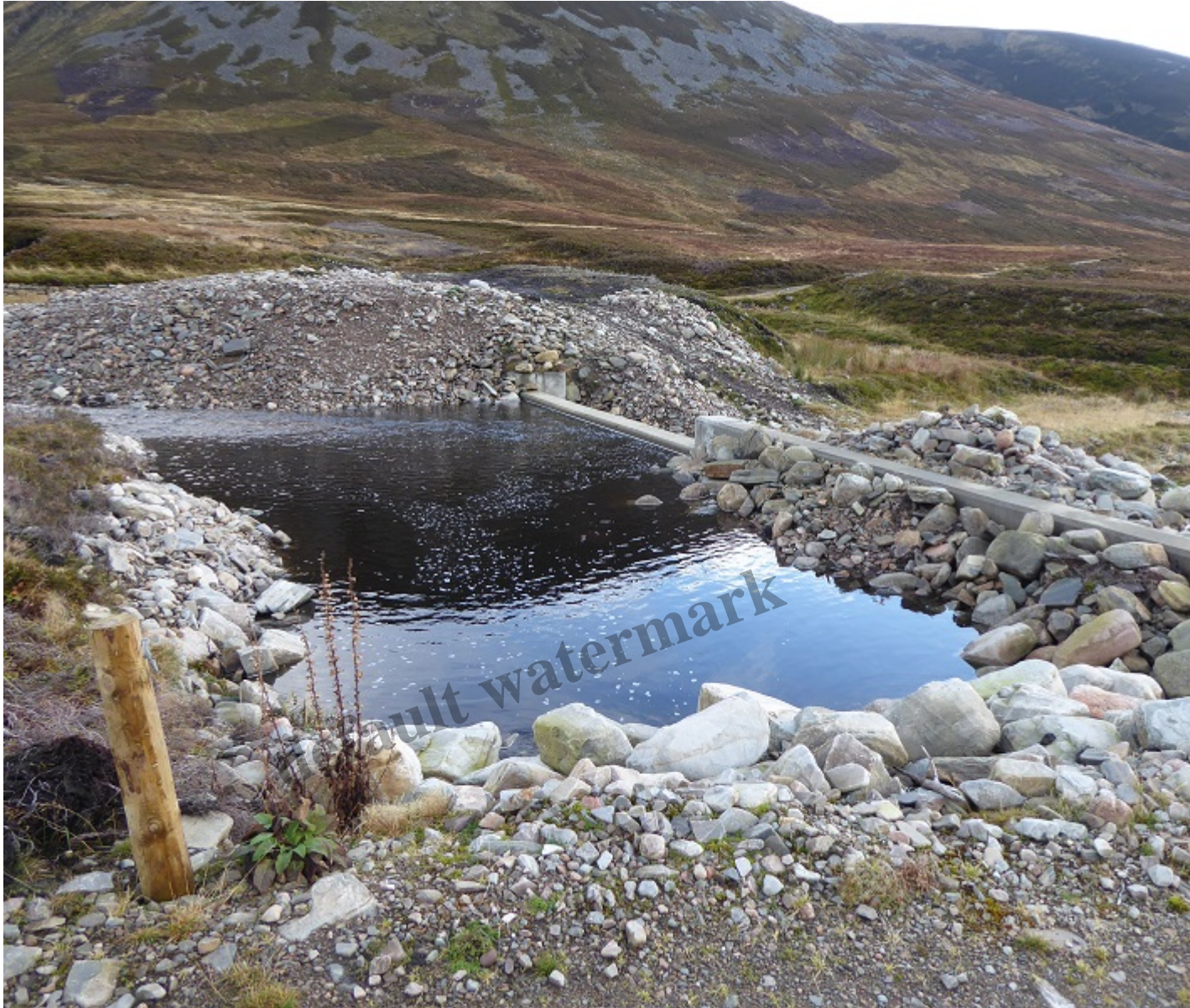
A pool was created at the secondary intake to make it appear more natural.
