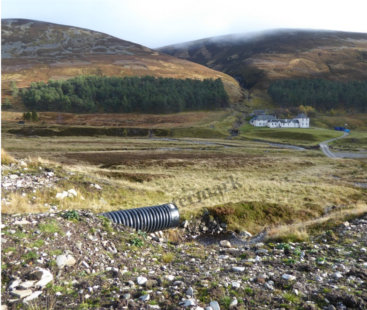
The worst of the protruding culverts
