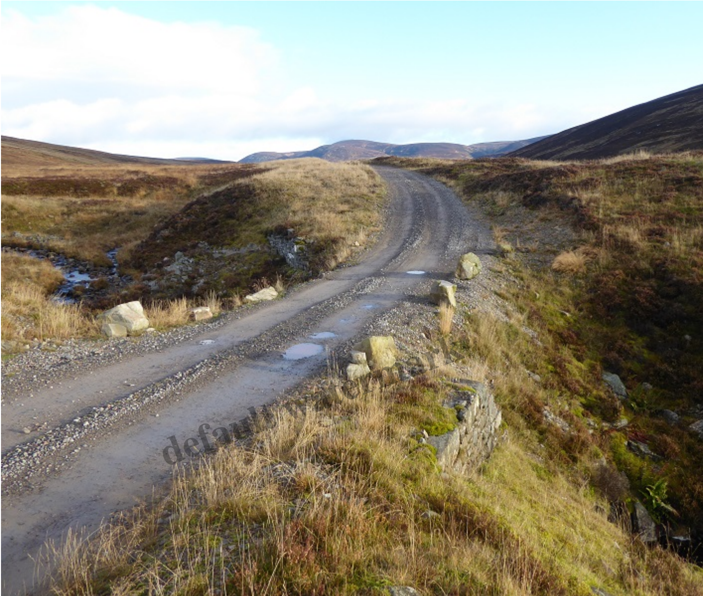
Poor finishing with material from the edge of the track spilling down towards the culverted burn below
