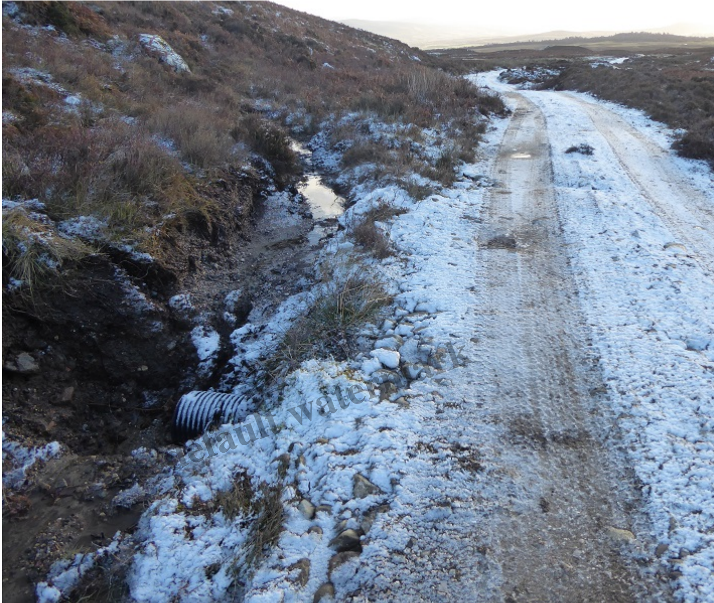
Unfinished culvert and new drainage ditch
