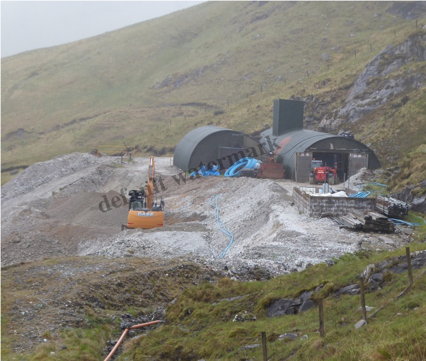
The Cononish gold mine as it looked on a dreich day in May – the same day as the pre-consultation Tyndrum Village Hall
