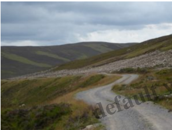
Looking south at the worst section of pipeline scar 2016
