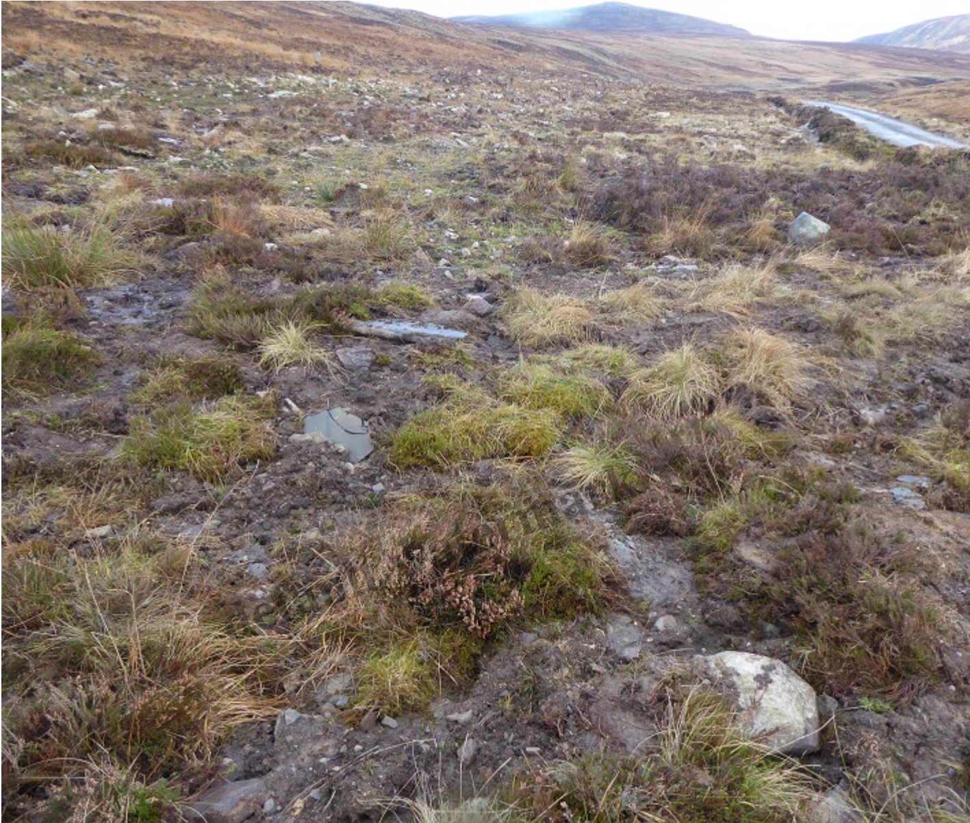
Restored boulder band scar showing how “robbed” turves and soil have been used.
