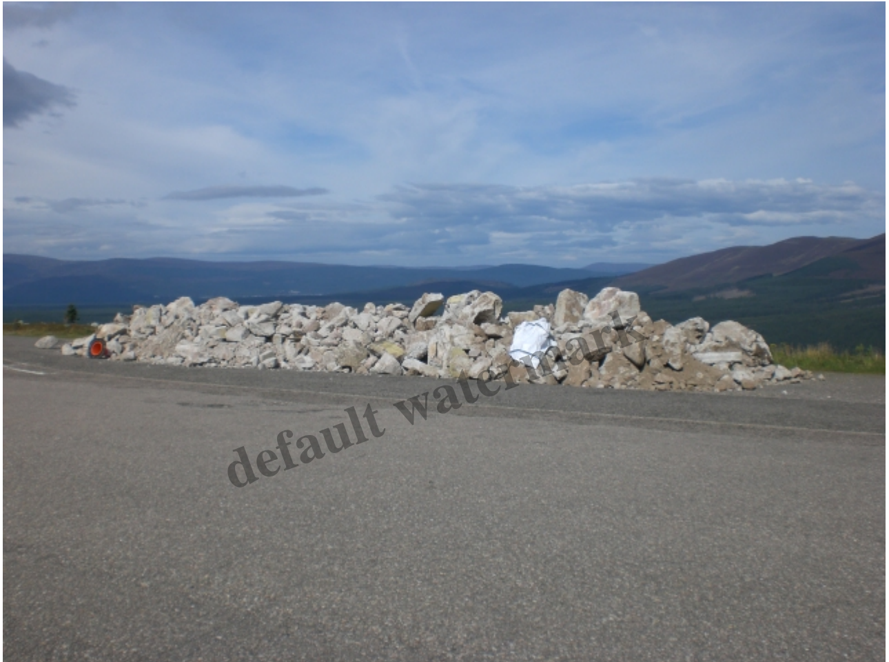
The concrete foundations of ski tows removed by truck from Coire na Ciste
