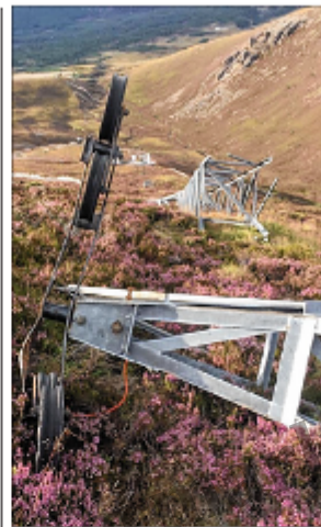
COIRE NA CISTE: Toppled lift towers.
