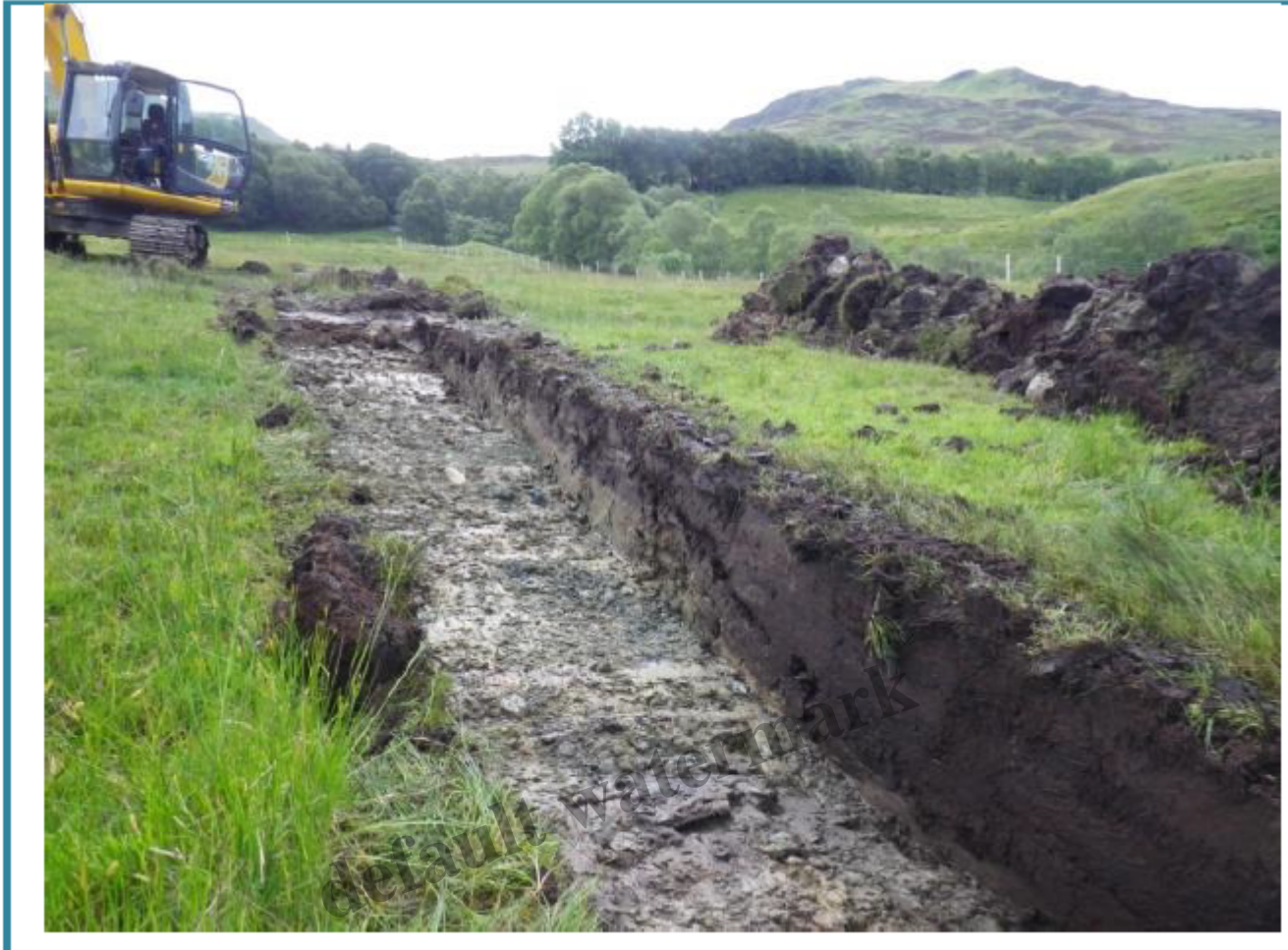
Photo from report of site visits in August 2015 at initial stage of construction
