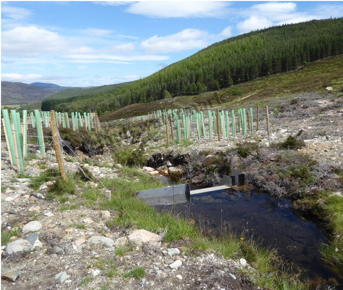
The small second intake, the pipe runs to the right of the blocks of trees which have been planted.
