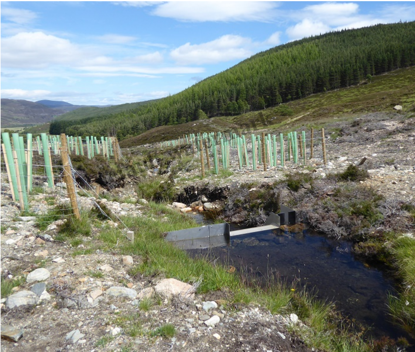
The small second intake, the pipe runs to the right of the blocks of trees which have been planted.
