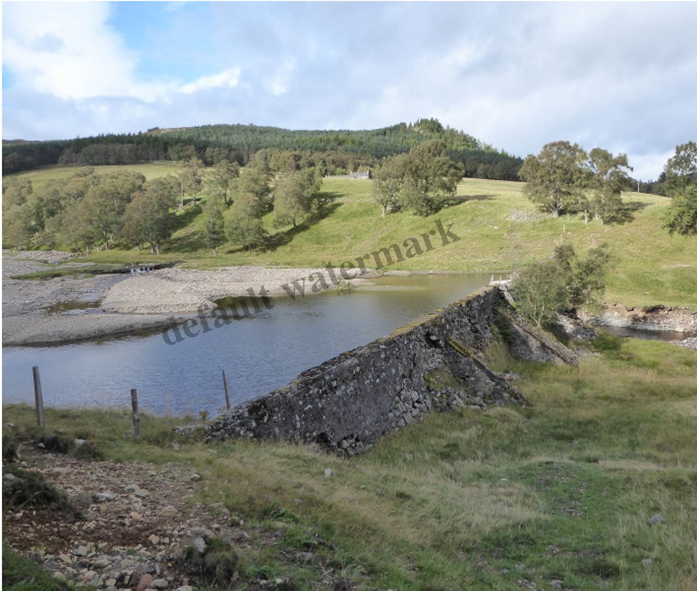
The old intake dam has been infilled with flood debris. You can just see old intake pipe centre left.
