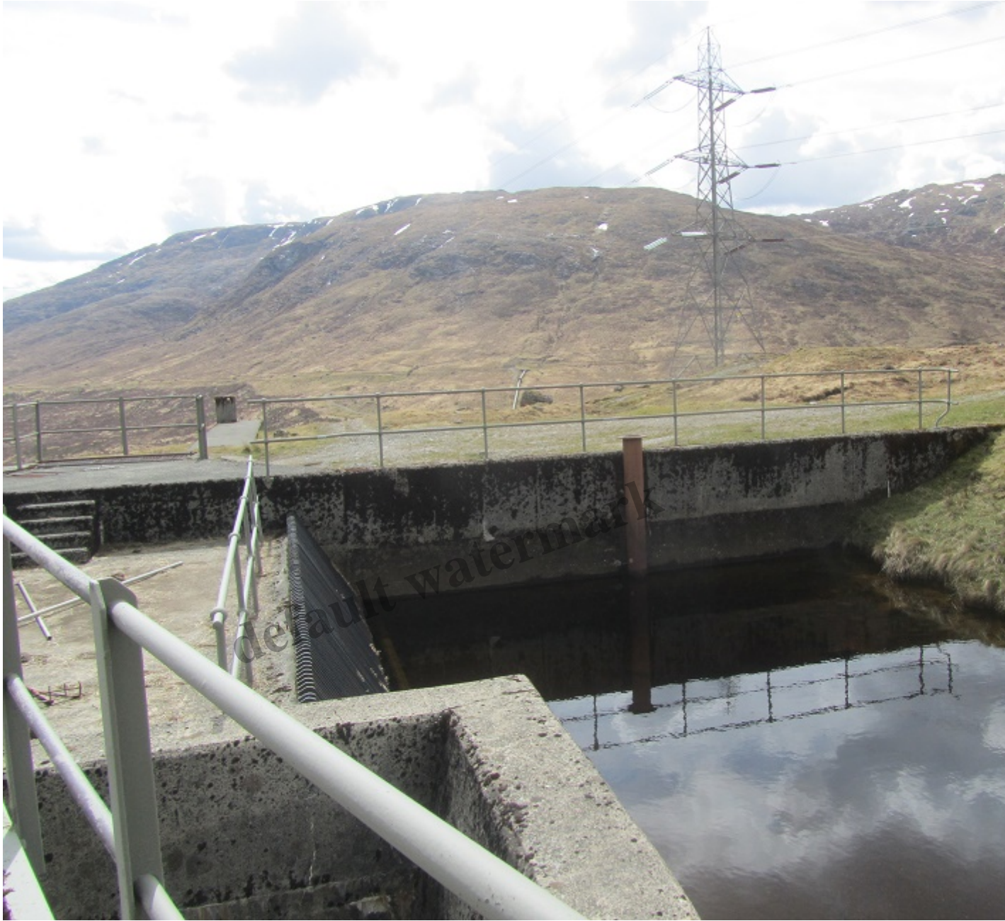
Alt nan Caoran Hydro intake south of Ben Lui and Ben Oss – you can just see pipeline above centre
