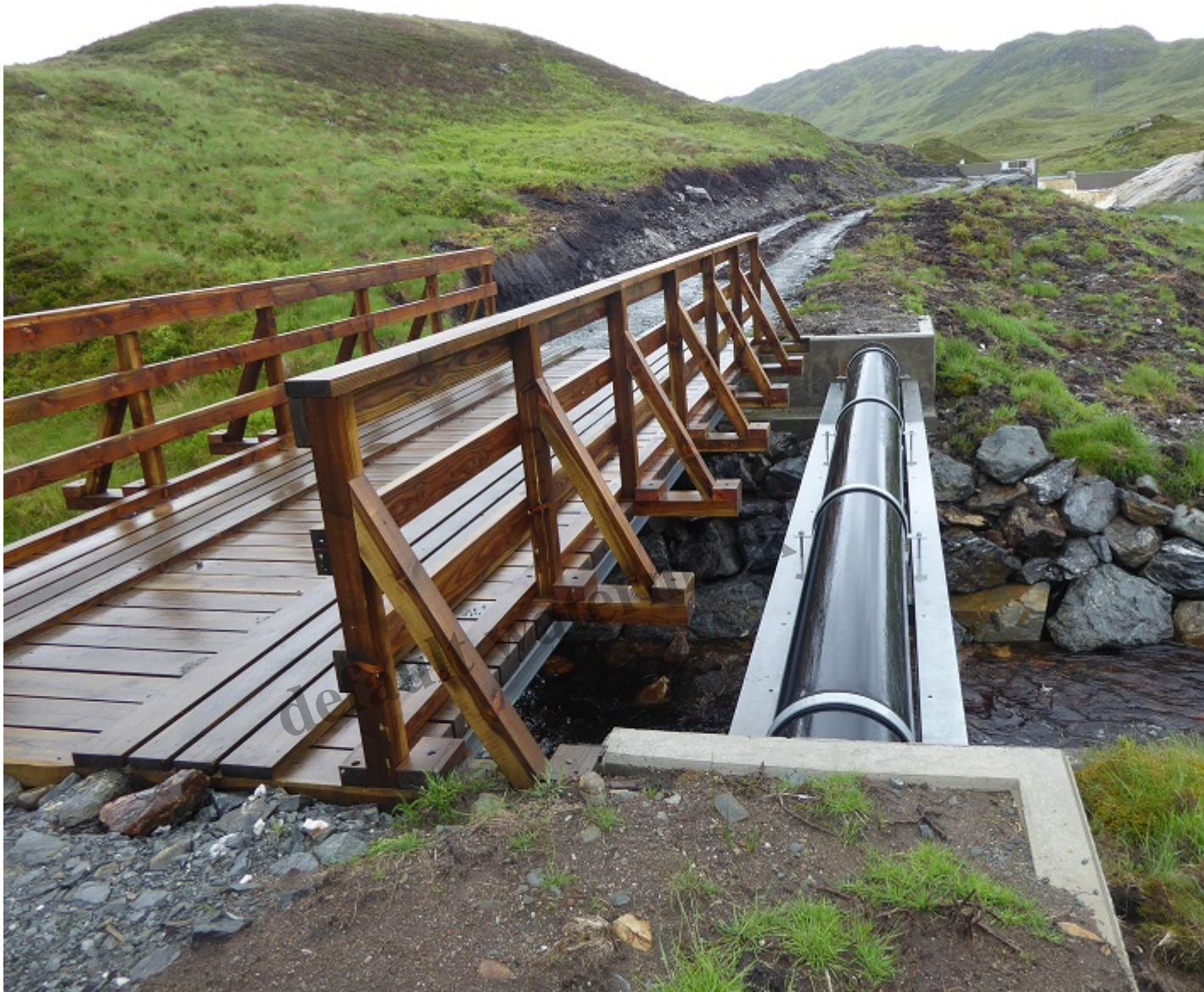
Beinn Ghlas hydro scheme – the LLTNPA appears uninterested in evaluating the impact of channeling the hill through pipes
