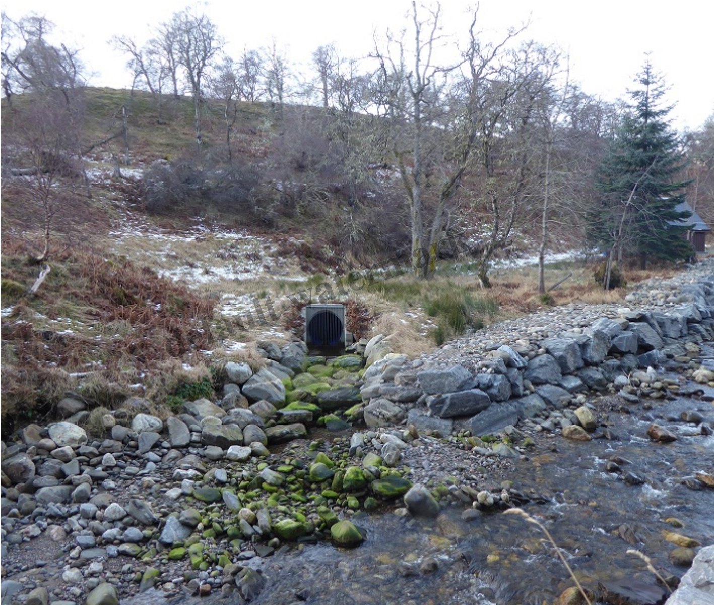
View from east side River Gynack of tailrace and powerhouse. The rip rap bouldering along the river the hydro scheme.
