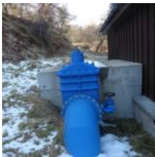
Close up of penstock
