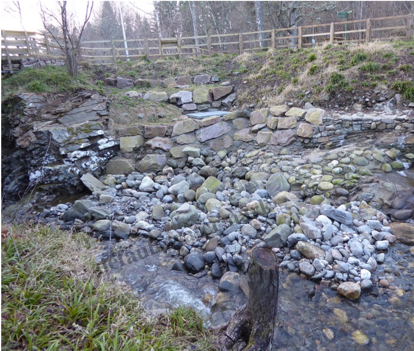
The line of the pipe, viewed from close to the intake, runs behind the line of the wall on the right.
