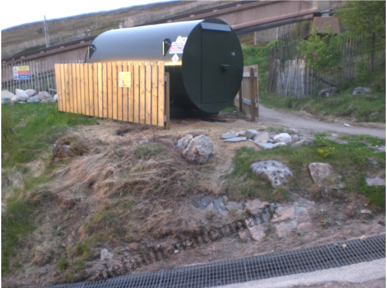
Diesel tank adjacent to funicular station – note dead vegetation centre and left
