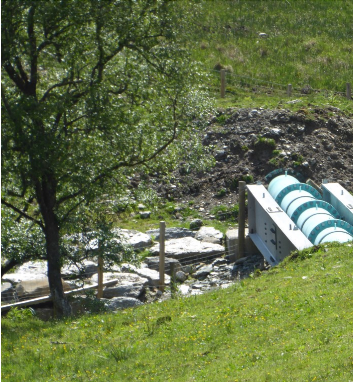
Penstock crossing Falloch between two metal girders – photo taken from just below A82
