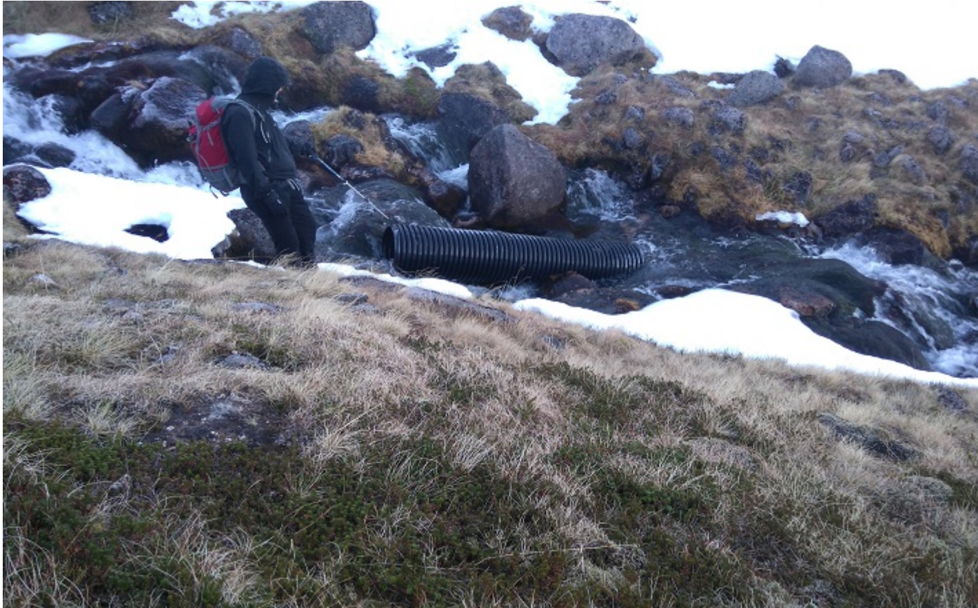
Windblown? pipe January 2017 Photo Credit Louis Mullen
