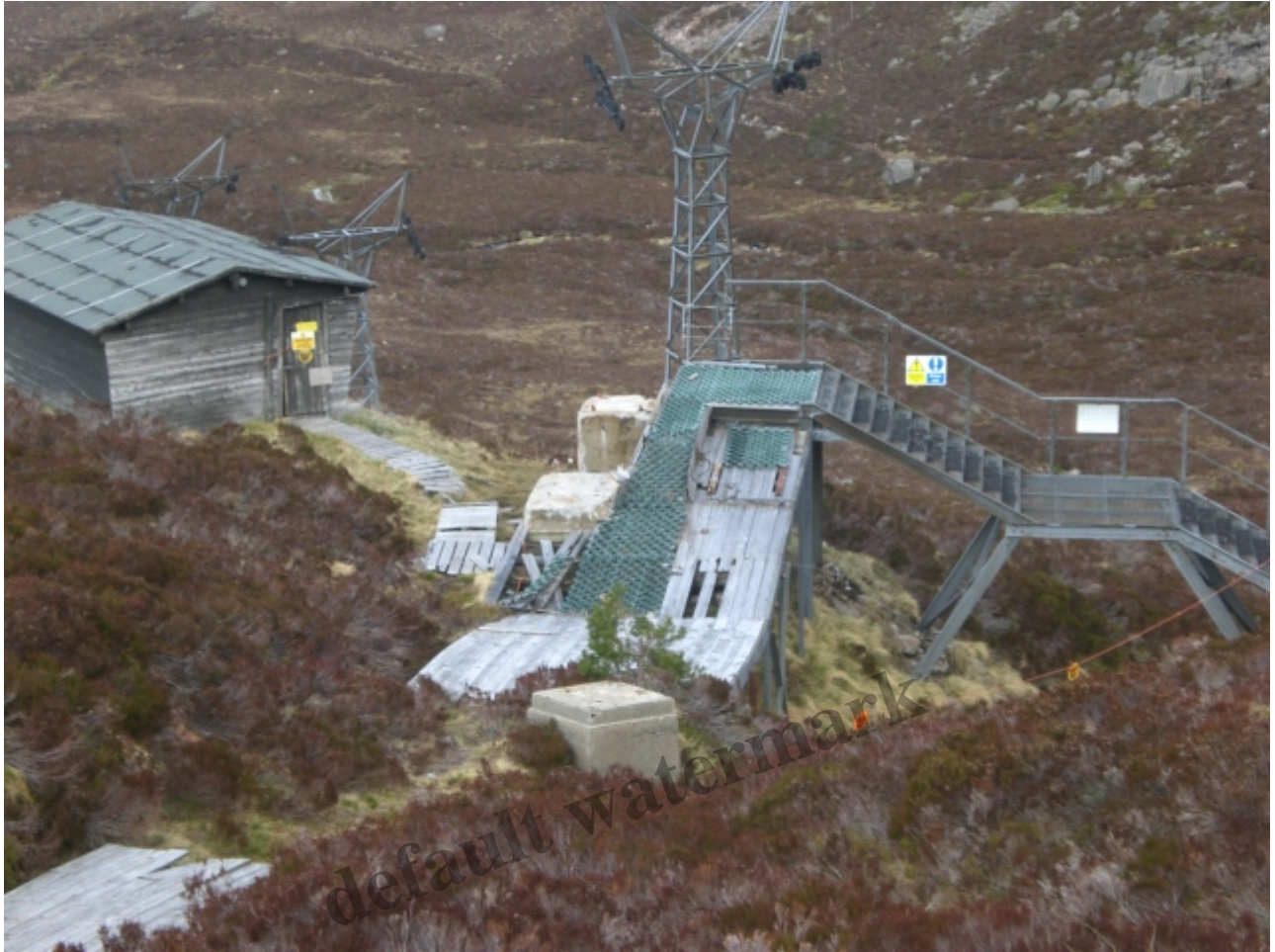
The Aonach Poma loading gantry – its been in this state for almost 7 years now
